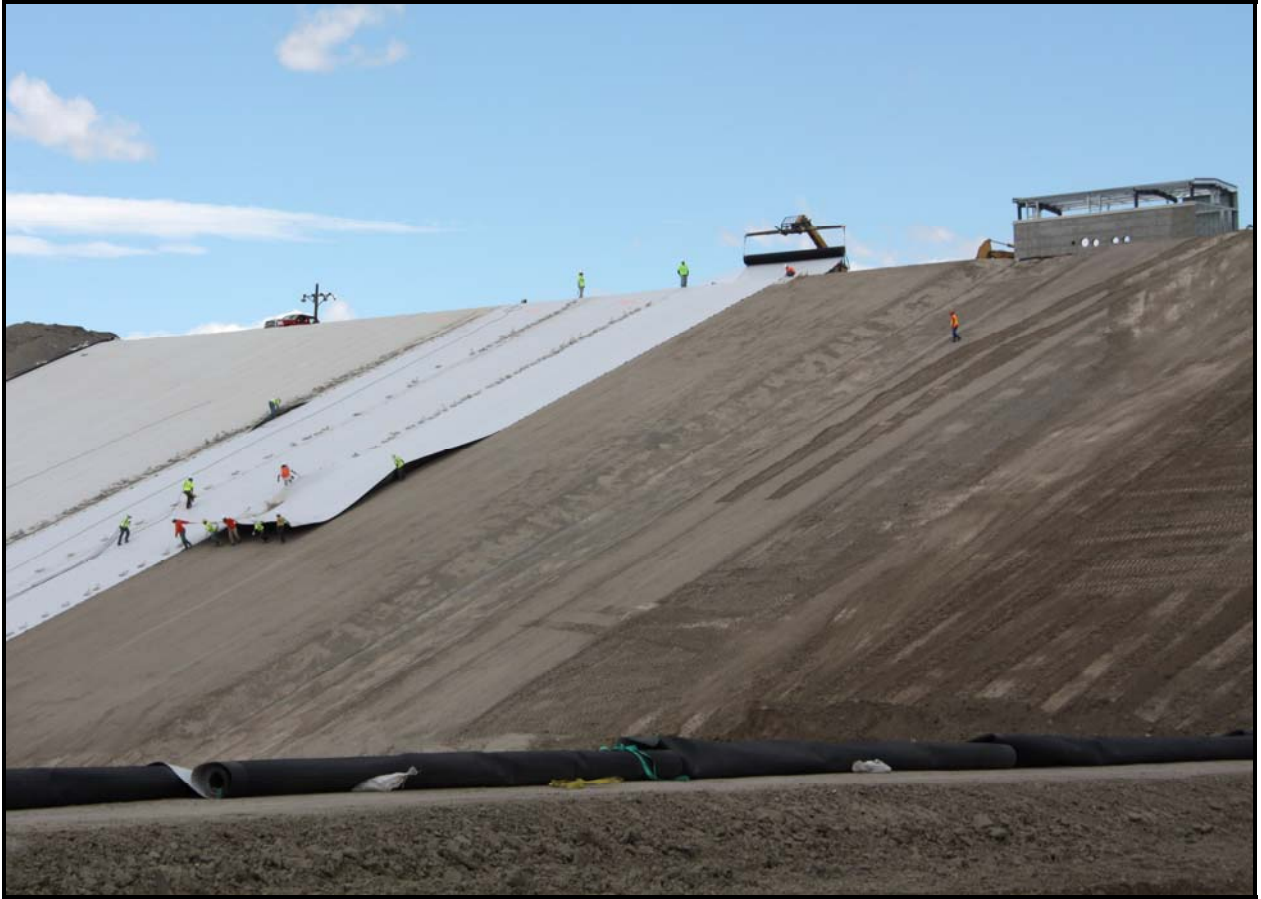
TradeWind Services/DelHur Industries personnel install the secondary high-density polyethylene liner on the north slope of super cell 9 at the Environmental Restoration Disposal Facility.
