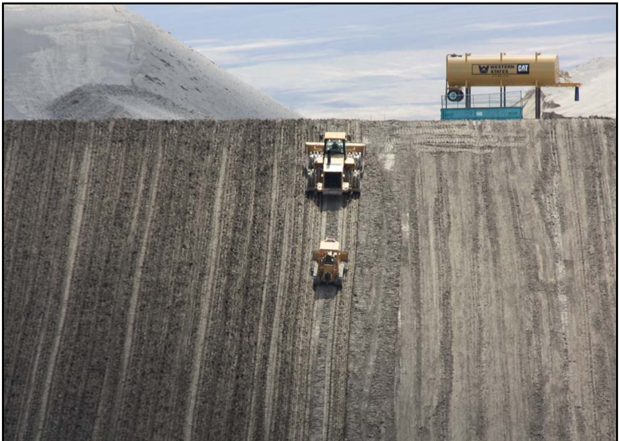
TradeWind Services/DelHur Industries personnel place admix on the south slope of super cell 10 at the Environmental Restoration Disposal Facility.
