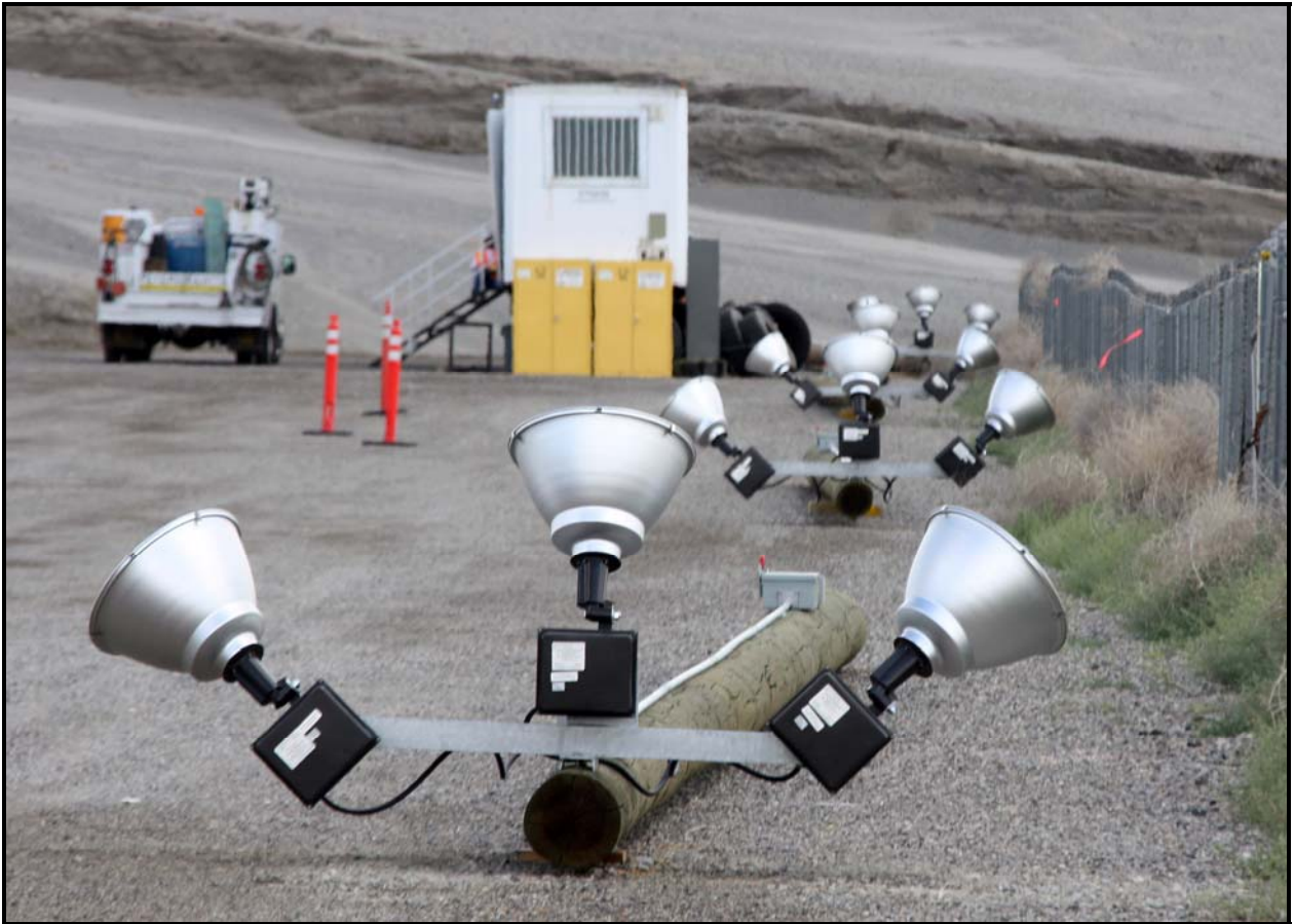
WCH subcontractor George A. Grant began installing light posts at the Environmental Restoration Disposal Facility's transportation yard.
