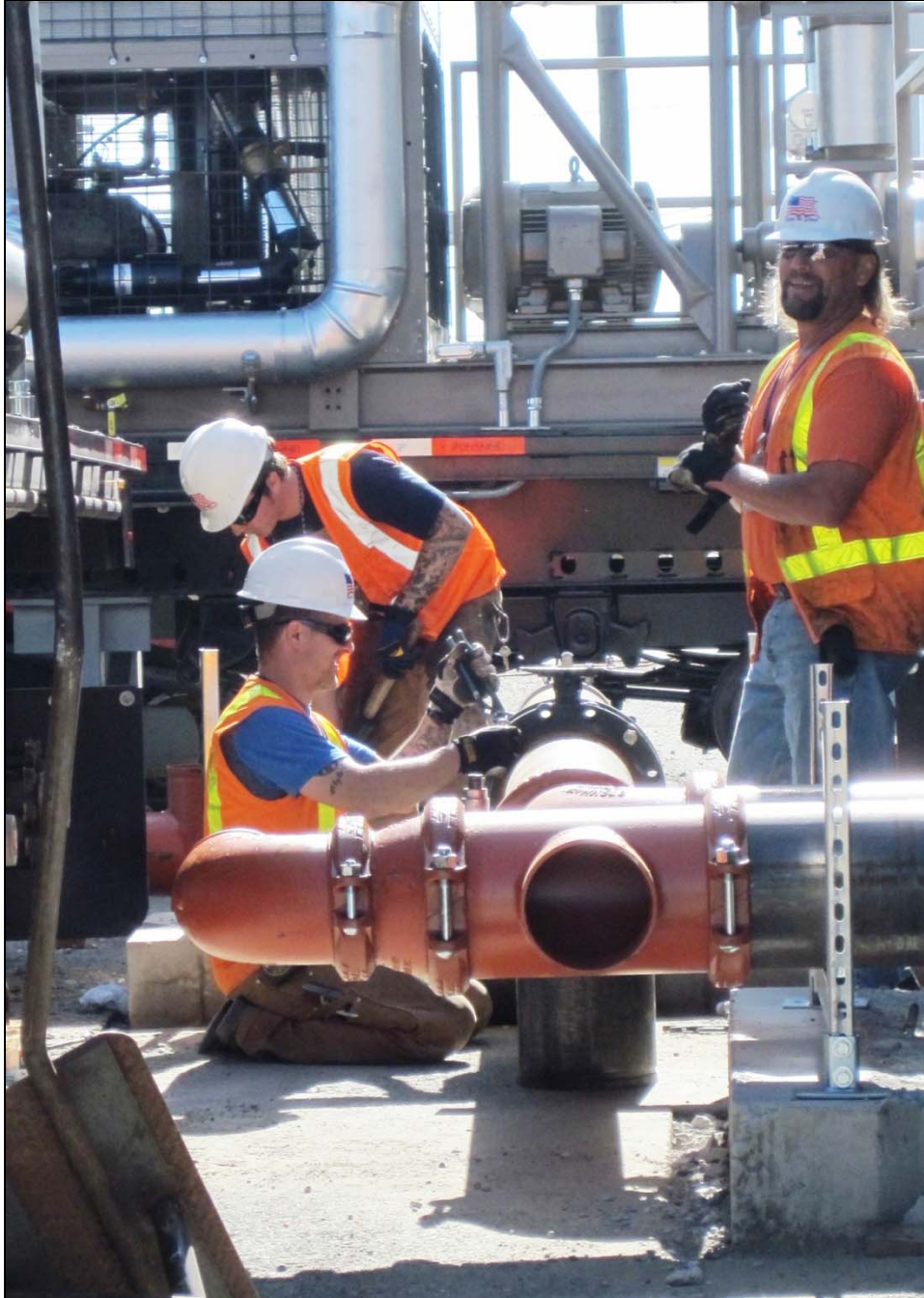
Workers install components for a chiller system that is being installed to improve working conditions at the Plutonium Finishing Plant
