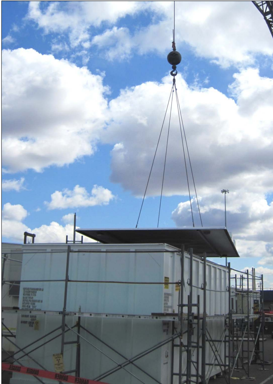
A lid is lowered onto a container of glove boxes and laboratory hoods removed from the 234-5Z building at the Plutonium Finishing Plant. The glove boxes and hoods were decontaminated to meet low-level waste criteria and the contents will now be shipped to and disposed of at the Environmental Restoration Disposal Facility.
