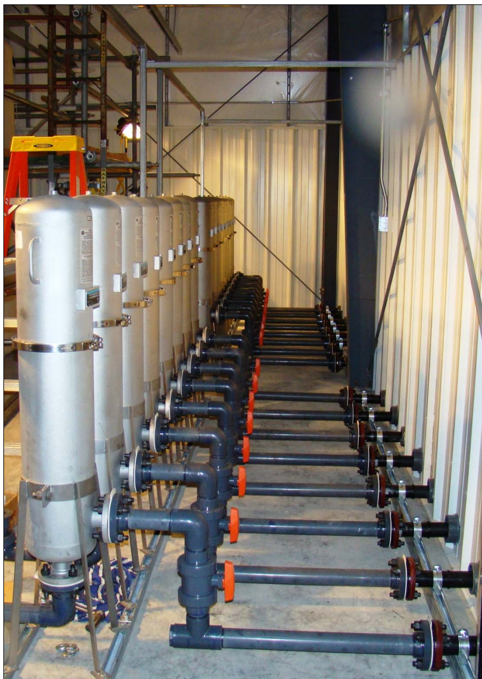
The interior of one of the DX transfer buildings, where equipment was recently installed to connect with piping that will carry water to and from the facility (see Photo 10).
