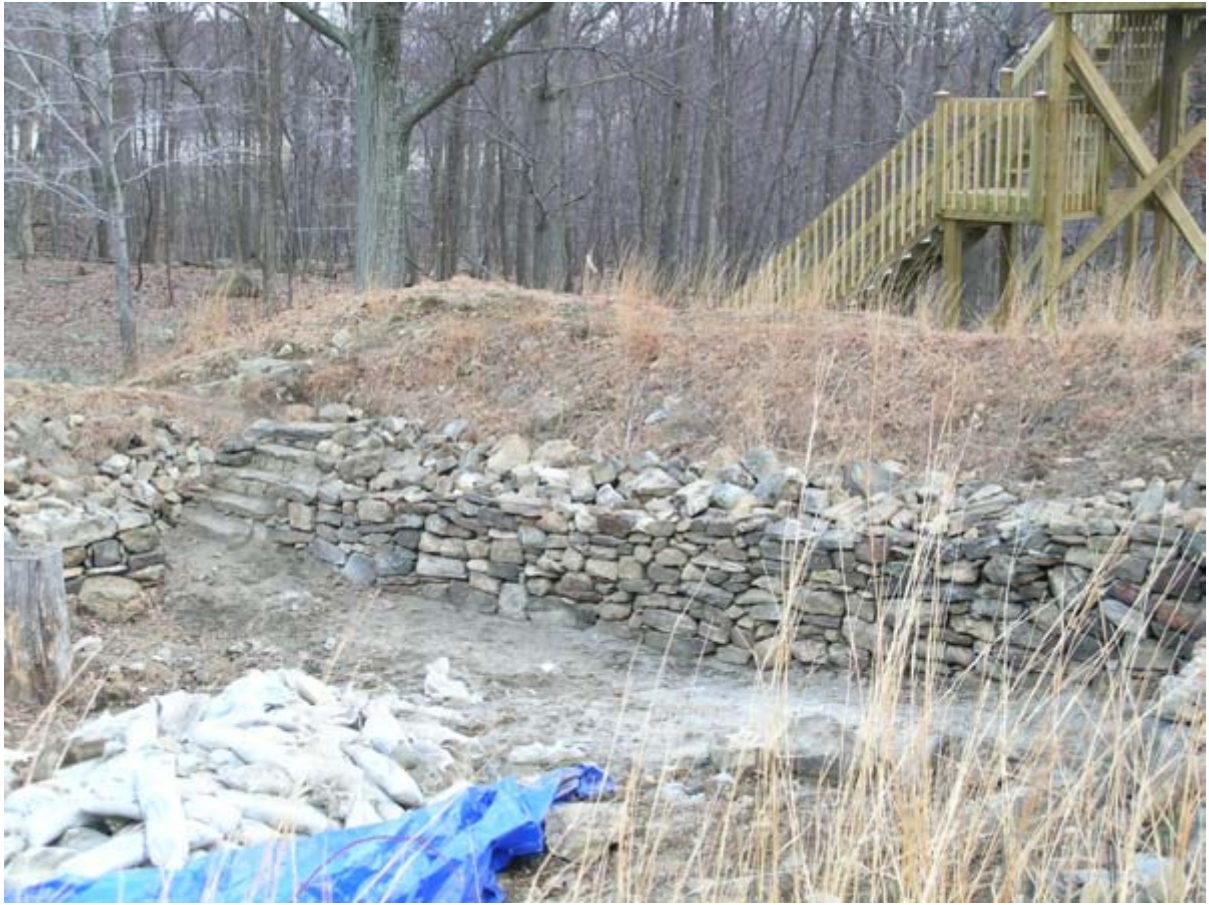
Stairs added to Interior of Redoubt No. 2, demonstration project. [D. Cubbison, January 2006]
