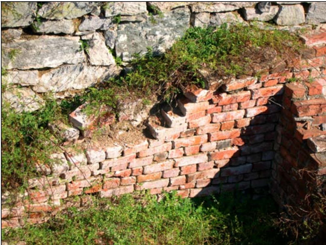
Photograph 31: Brick Collapse, Interior of Romans' Powder Magazine, Looking East. (D. R. Cubbison, 31 October 2003)
