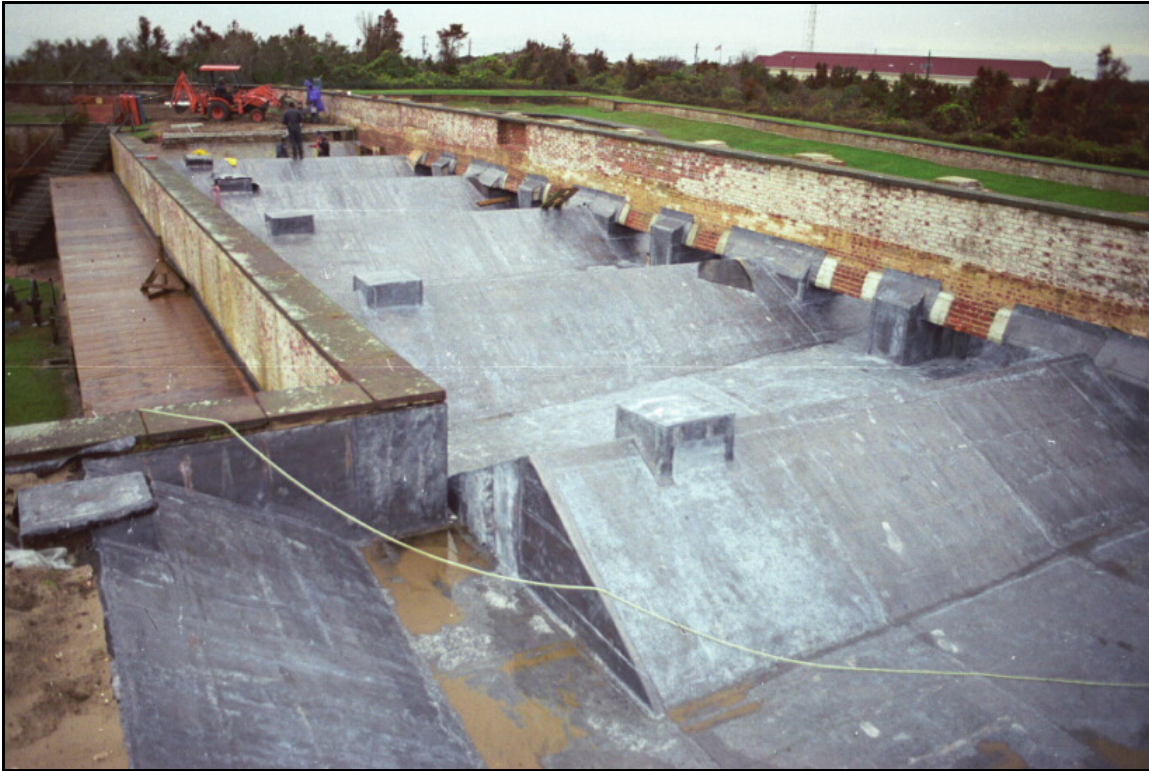
Photograph 42: View looking at the excavated casemates at Fort Macon, North Carolina. The design of the gutter system is similar to the system at Fort Monroe, Virginia. The major difference is that the Fort Macon Casemates are constructed of lead coated copper covered with tar while the Fort Monroe Casemates are ceramic tiles coated with tar.
