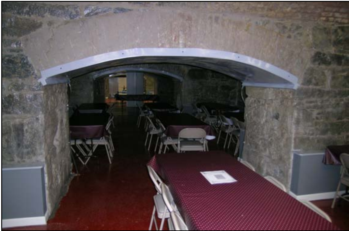
Photograph 45: Interior view of Casemate 21 of the arches that provide access between the vaults. Water is seeping through the masonry and collecting on the floor of the vaults, also a recurring problem in Casemates 20 and 22. In the 1990s, engineers installed a water collection system intended to drain the water. While this has been marginally effective at preventing water from pooling, it does not solve the cause of the problem, which is the failure of the gutter system.
