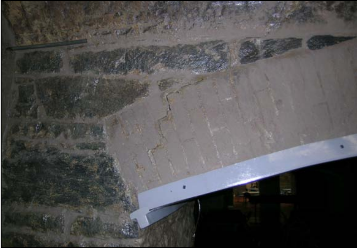
Photograph 47: Detailed view of one of the arches in Casemate 21. The mortar in this arch failed and a crack has developed in the arch, which has likely compromised its structural integrity. Note the glossy surface of the stone. At some point, a coating was applied to the masonry to control dust. This coating may be contributing to the deterioration of the mortar as it serves to trap moisture in the walls.
