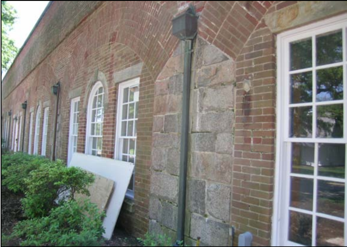
Photograph 40: Detailed view of one of the exterior gutters at Casemate 21. These gutters provide an outlet for the moisture that is collected by the gutter system. A cursory inspection of these gutters indicates that at least some water is flowing out of the downspouts. This indicates that a portion of the drainage capability of the gutter system is intact. Note that some of the mortar exhibits signs of biological growth, and that several of the mortar joints have failed.
