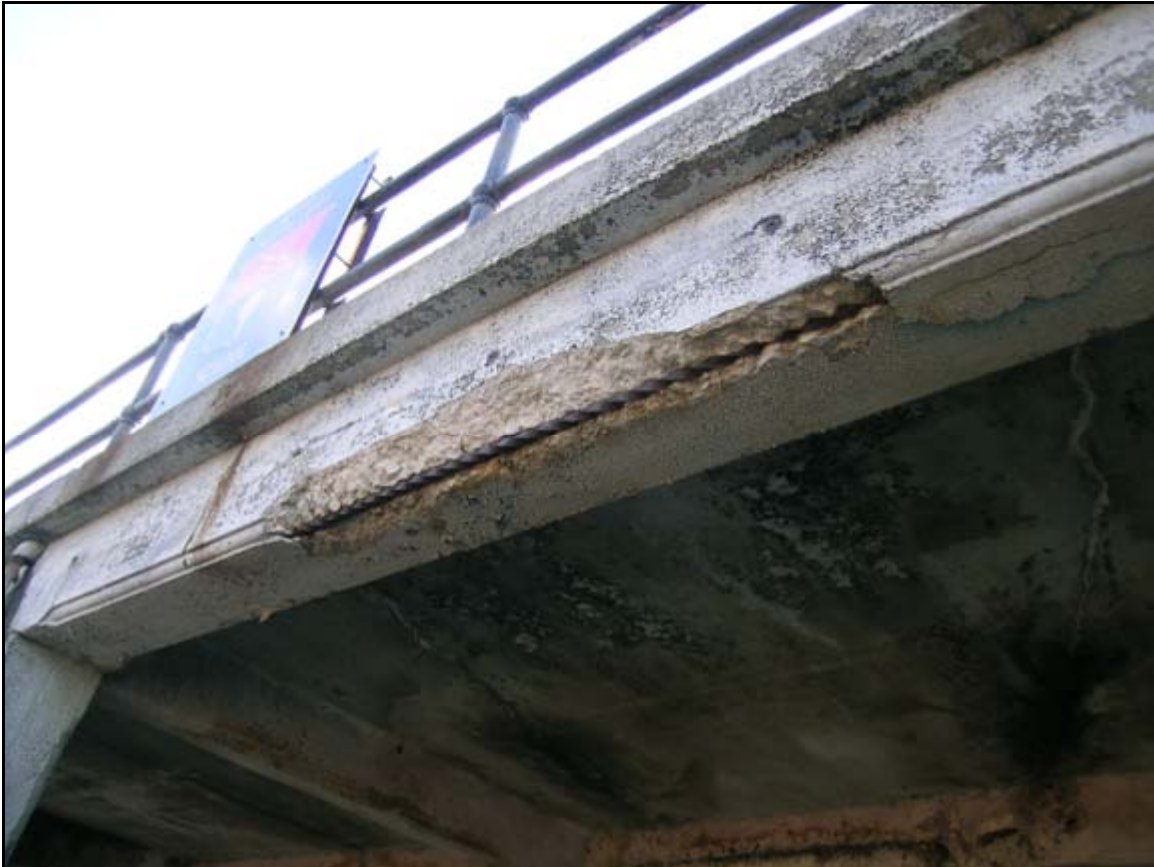
Photograph 5: View looking at Battery DeRussy, Fort Monroe, Virginia. This particular portion of the concrete spalled off and exposed the steel reinforcement beam embedded in the concrete. This condition may have occurred as a result of salts in the concrete rusting the steel. When steel corrodes it expands, which in turn caused the concrete face to spall off the building
