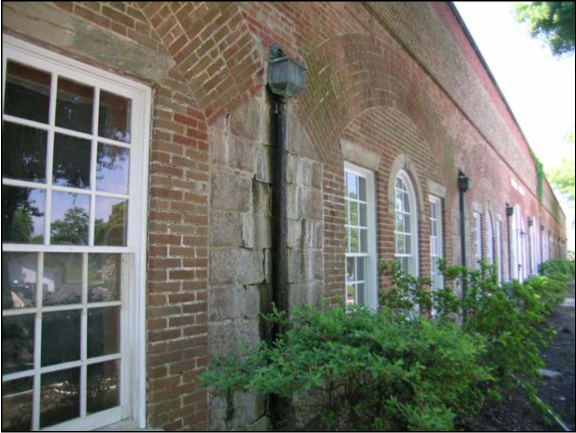
Photograph 41: View looking at another gutter on the exterior of Casemate 21. Although this appears to be functioning, the presence of efflorescence around the gutter and on the masonry indicates that moisture is seeping out through the masonry and depositing salts on the brick exterior. This suggests that the interior gutter system has at least partially failed.
