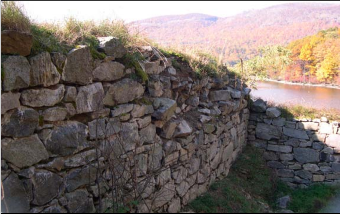
Photograph 30: Catastrophic Failure, sixty square foot collapse, Interior of Romans' Powder Magazine, Looking North. (D. R. Cubbison, 31 October 2003)
