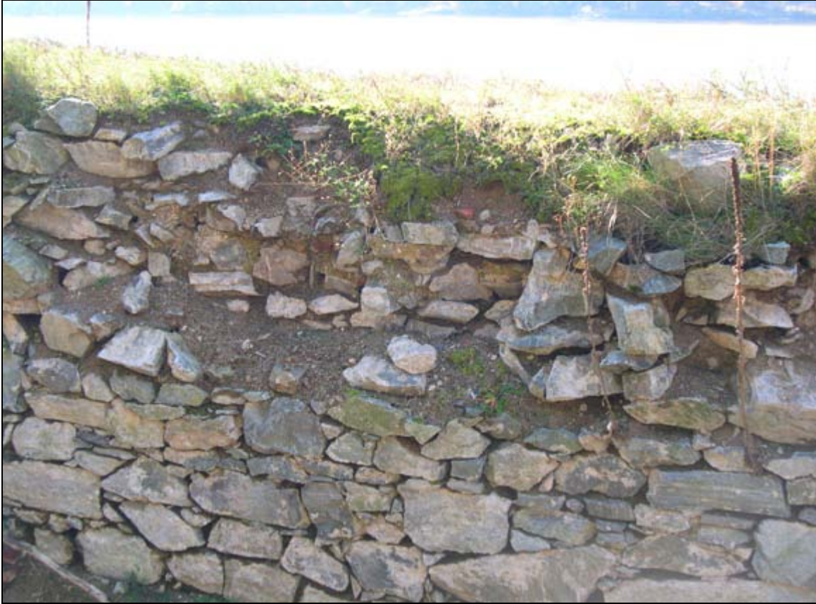
Photograph 28: Catastrophic Failure, sixty square foot collapse, Interior of Romans' Powder Magazine. (D. R. Cubbison, 31 October 2003)
