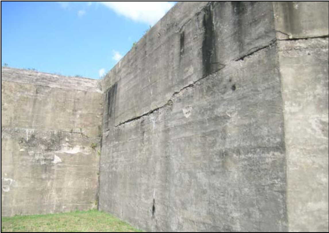
Photograph 3: View looking at the seaward side of Battery DeRussy at Fort Monroe, VA. Note the horizontal crack on this exterior wall. This is an example of a cold joint, a condition that occurs when a layer of concrete is poured adjacent to a layer that has been allowed to harden. Cracks such as these allow moisture to infiltrate the structure and cause a great deal of damage. Note the presence of biological growth in some of cracks; this is a clear sign that moisture is present within the exterior walls. This portion of Battery DeRussy was once covered with earth but it was removed in the 1950s to accommodate base housing.
