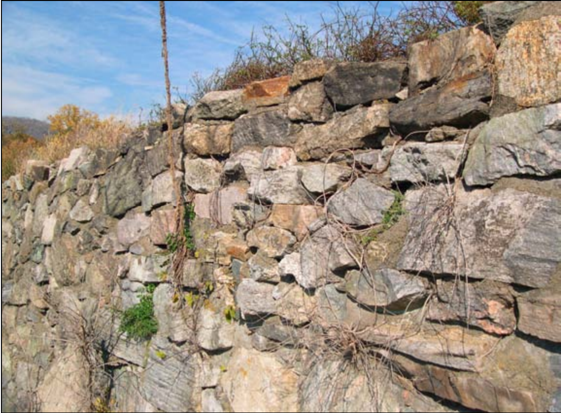
Photograph 34: Imminent Failure of Exterior Masonry Parapet Wall, Romans' Powder Magazine. (D. R. Cubbison, 31 October 2003)
