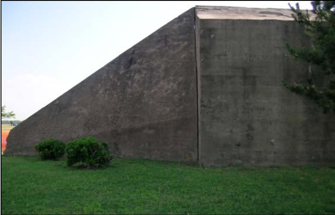
Photograph 4: View looking at Battery Church, Fort Monroe, Virginia. These particular sections have completely separated from each other. This may be a result of the use of a plane of weakness in the original design of the battery. A plane of weakness creates a joint between two adjacent sections of concrete that is designed to fail. This allows engineers to prevent unwanted cracks in concrete structures by allowing sections to settle independently of each other.
