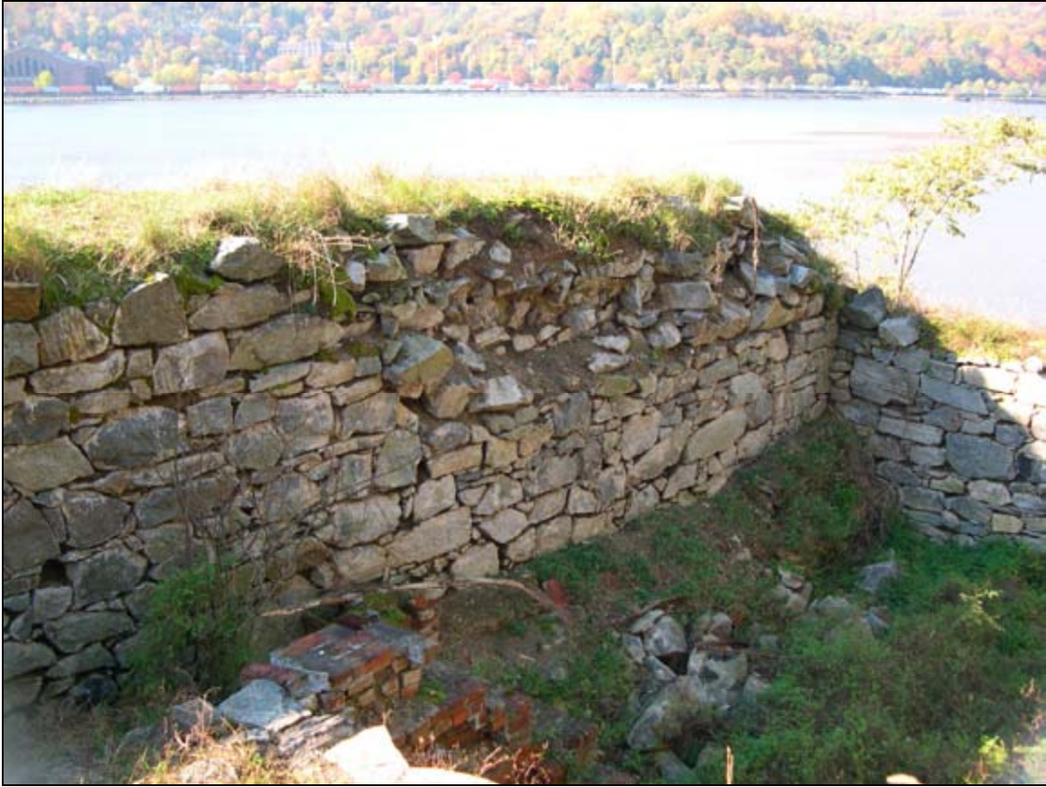
Photograph 27: Catastrophic Failure, sixty square foot collapse, Interior of Romans' Powder Magazine, Looking Northwest.
