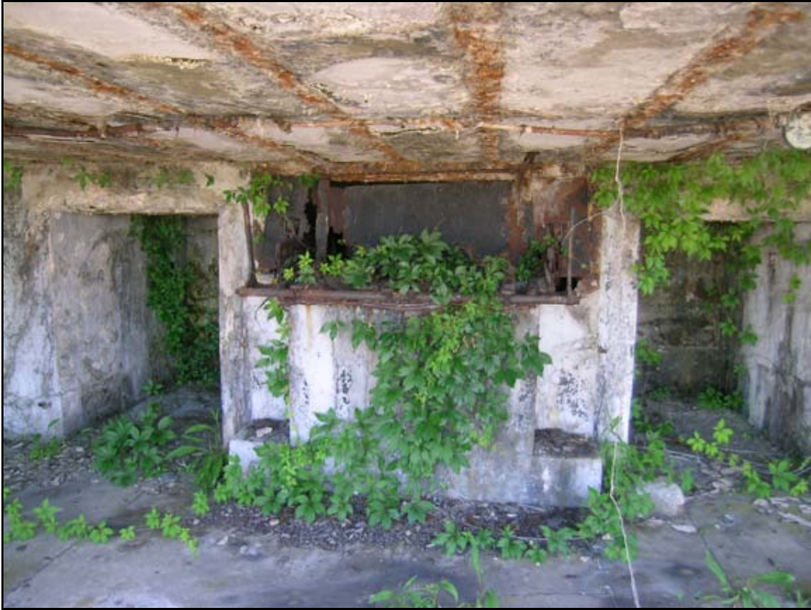
Photograph 10: View looking at one of the chain hoist system at Battery DeRussy, Fort Monroe, Virginia. The presence of substantial biological growth, extensive corrosion, and the great amount of spalling that has occurred indicates a significant amount of moisture infiltration. Before any rehabilitation work can begin, the building needs to be allowed to dry out. (Photograph by T. Beckwith, June 2005)
