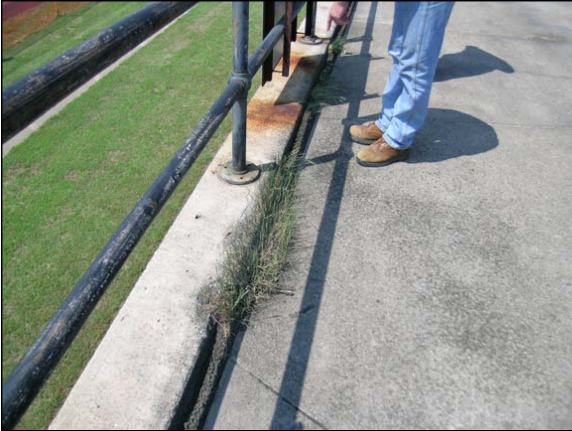
Photograph 2: View looking at the drainage gutter on the inland side of Battery DeRussy at Fort Monroe Virginia. Soil and debris completely filled in this gutter significantly affecting the ability of the structure to shed water during periods of precipitation.
