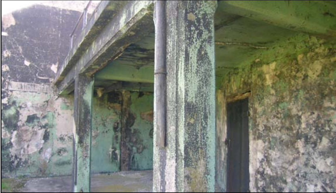
Photograph 11: Detailed view of one of the leaders at Battery Parrott, Fort Monroe, Virginia. Many of the downspouts and leaders are missing or severely damaged, which is the case with this particular example. This condition inhibits the drainage system's ability to guide water away from the foundation of the building.
