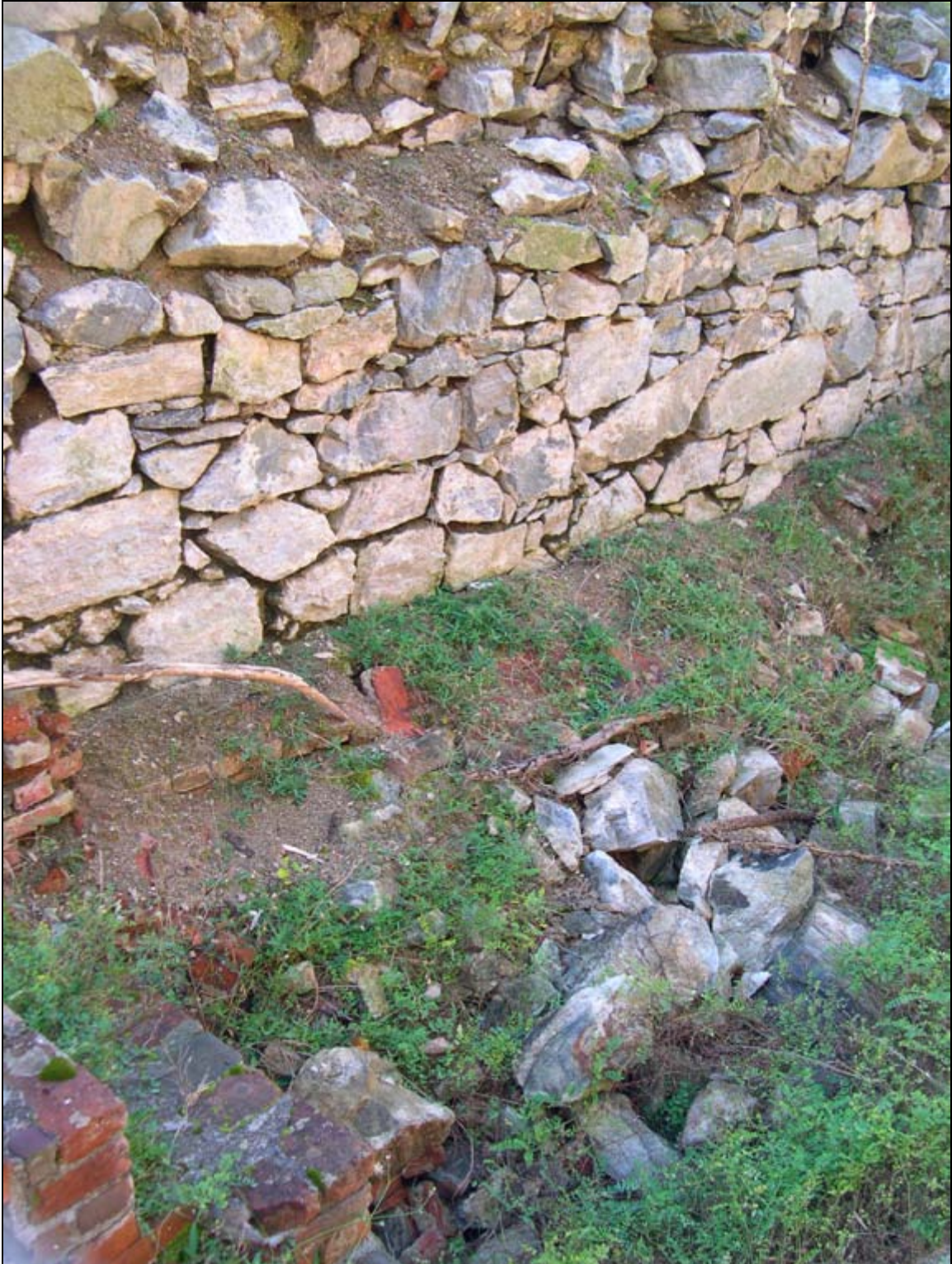
Photograph 29: Catastrophic Failure, sixty square foot collapse, Interior of Romans' Powder Magazine. (D. R. Cubbison, 31 October 2003)
