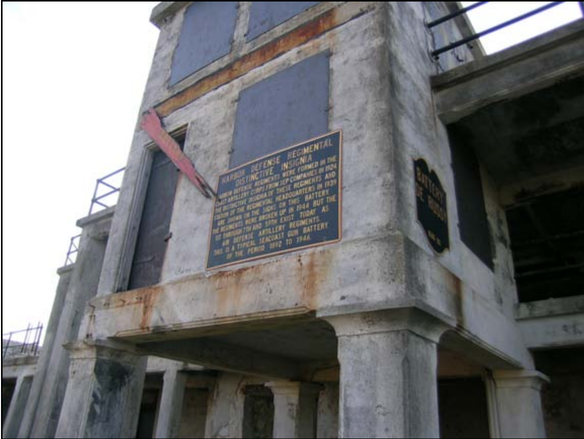
Photograph 9: View looking at Battery DeRussy, Fort Monroe, Virginia. These rust stains are likely a result of the metal stairs that once provided access to the tower. Discoloration such as these is generally cosmetic and does not pose a threat to the continued preservation of the structure. Stains however should be scrutinized to ensure that they are not caused by a more serious issue. (Photograph by T. Beckwith, June 2005).
