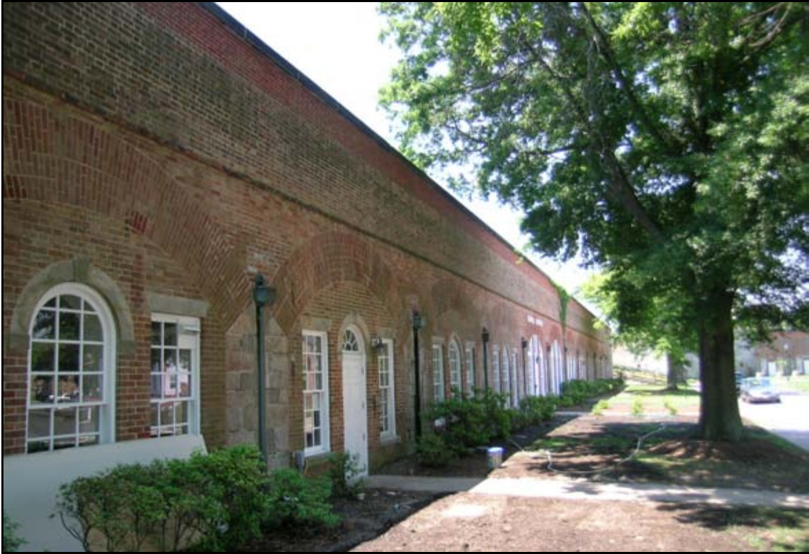
Photograph 38: View looking at the exterior of Casemate 21, Fort Monroe, Virginia. These exterior walls exhibit efflorescence around the gutter down spouts. Biological growth can also be discerned along the upper brick courses, another indication of moisture infiltration into the masonry walls. (Photograph by T. Beckwith, June 2005)
