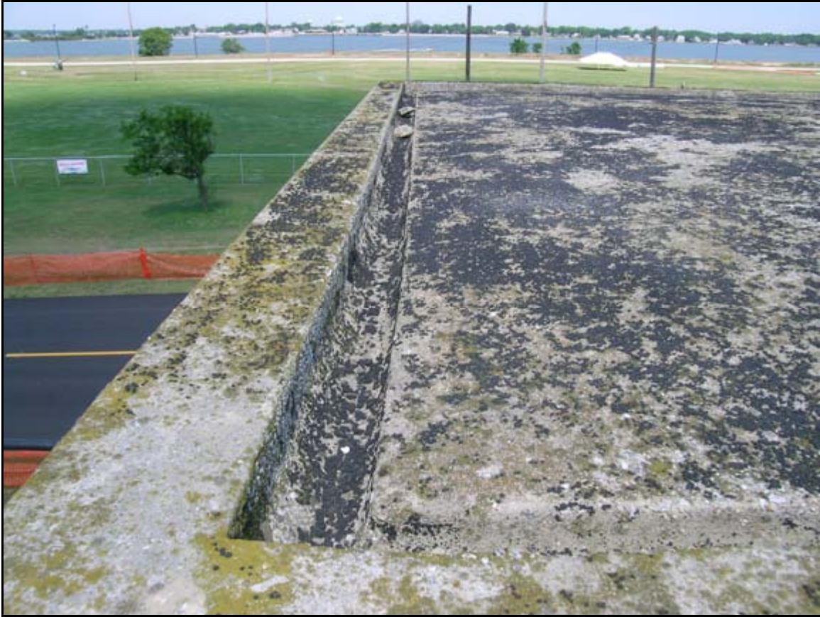
Photograph 7: View looking at the top of the observation tower, Battery DeRussy, Fort Monroe, Virginia. This tower exhibits some erosion caused by exposure to weather. Overtime, erosion will wear away the surface layer of concrete and ultimately allow moisture to infiltrate the structure. The black on the roof appears to be tar, which was routinely applied to waterproof the building. (Photograph by T. Beckwith, June 2005).
