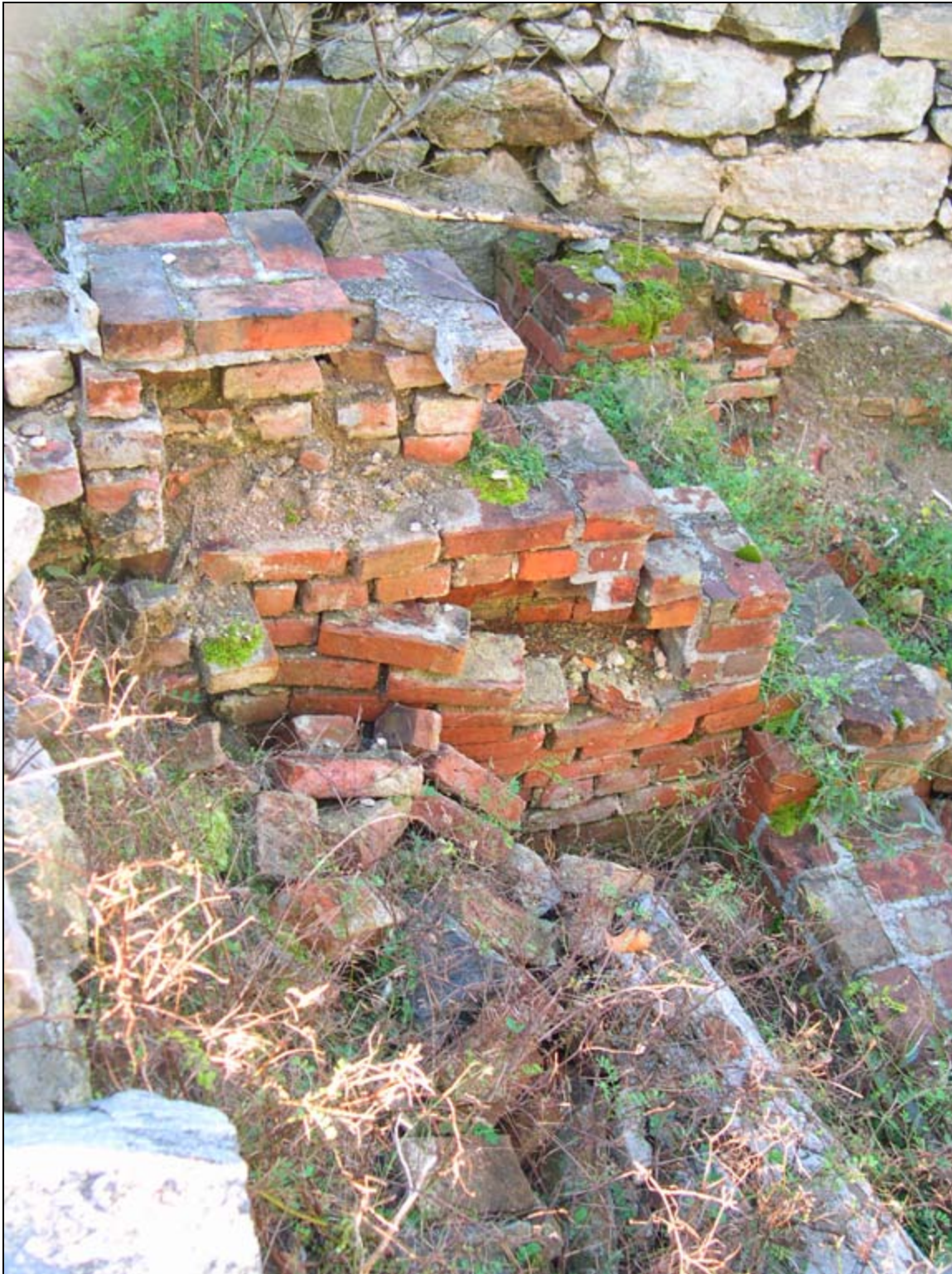
Photograph 32: Collapse of Brick Stairs, Interior of Romans' Powder Magazine, West Entrance. (D. R. Cubbison, 31 October 2003)
