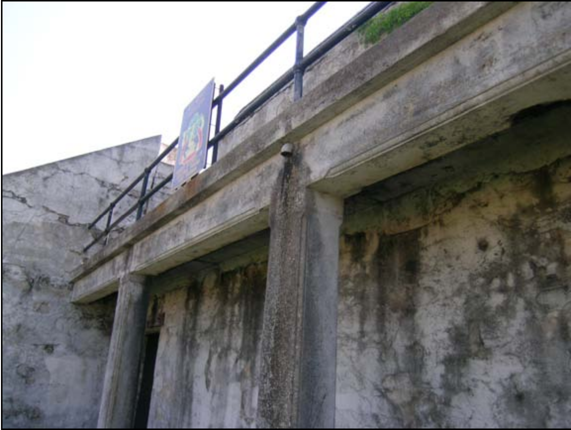
Photograph 6: View looking at Battery DeRussy, Fort Monroe, Virginia. This portion of the battery exhibits a number of cracks with varying degrees of severity. Most of these are superficial but should be monitored over time to ensure that they are not adversely affecting the structural stability or allowing moisture to infiltrate the walls. Note that the two leaders and downspouts in the center of the photograph have been entirely removed.
