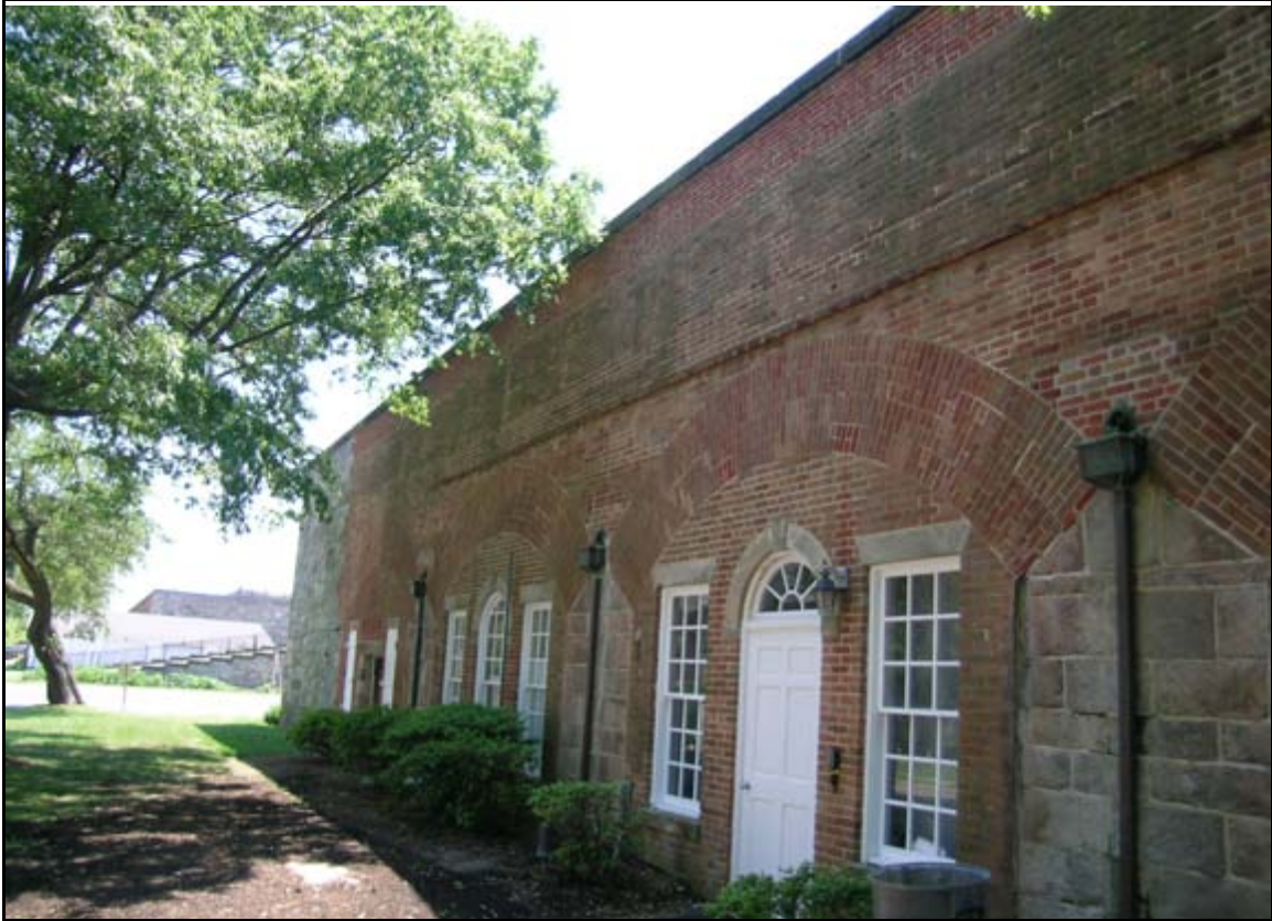
Photograph 39: View looking at the exterior of Casemate 21, Fort Monroe. This casemate suffers from extensive moisture infiltration. The failure of the gutter system or the membrane that covers each of the arches allowed moisture to penetrate the structure. Note that portions of this brick wall have been re-pointed. It is unclear if an appropriate mortar mixture was used in this re-pointing of the masonry walls. (Photograph by T. Beckwith, June 2005)
