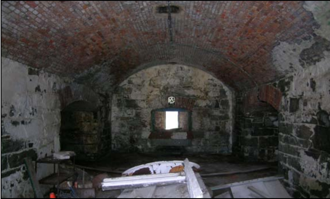
Photograph 43: View looking at one of the vaults in Casemate 22, Fort Monroe, Virginia. This arch exhibits signs of significant moisture infiltration; the most obvious is the amount of efflorescence on the surface of the masonry. Over time, the moisture in the walls will cause the mortar joints to fail. Left untreated, this condition will persist and the structural stability of the casemate will be compromised. (Photograph by T. Beckwith, June 2005)
