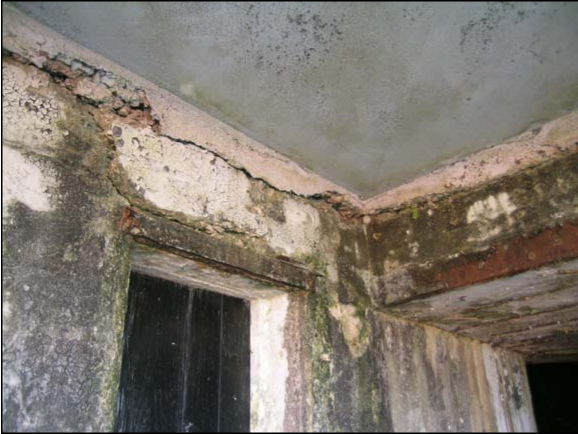
Photograph 8: Detailed view looking at the underside of Battery DeRussy, Fort Monroe, Virginia. This portion of the wall exhibits significant spalling. Spalling can occur for many reasons, in this instance it appears that moisture infiltrated the concrete walls causing the surface layer to fall off. This portion of the building also features a substantial amount of biological growth, clear evidence of a serious moisture problem.
