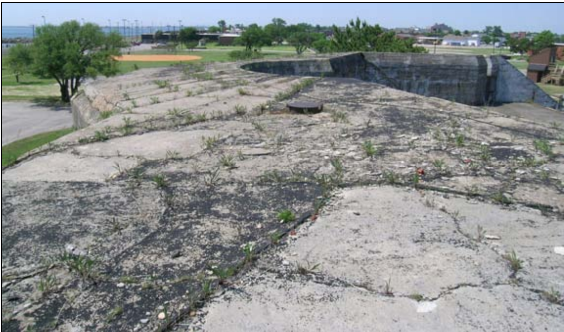
Photograph 14: View looking at the roof of Battery DeRussy, Fort Monroe, Virginia. The low pitch of the roof makes it difficult for the structure to shed moisture during periods of high precipitation. Engineers recognized the need for a working drainage system, and stipulated that the gutters, downspouts, and drains be cleaned on a weekly basis. The black substance appears to be tar or asphalt, which was applied to keep moisture from infiltrating the battery. This coating failed and the roof is now exhibiting some cracking. The presence of biological growth in the cracks clearly indicates a significant amount of moisture infiltration into the concrete.
