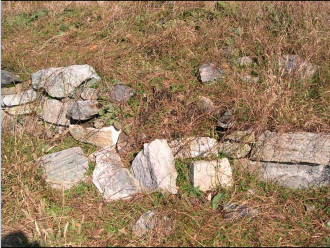
Photograph 35: Six Square Foot Collapse, Romans' Battery Parapet (Scarp) Wall, South of Romans' Powder Magazine. (D. R. Cubbison, 31 October 2003)
