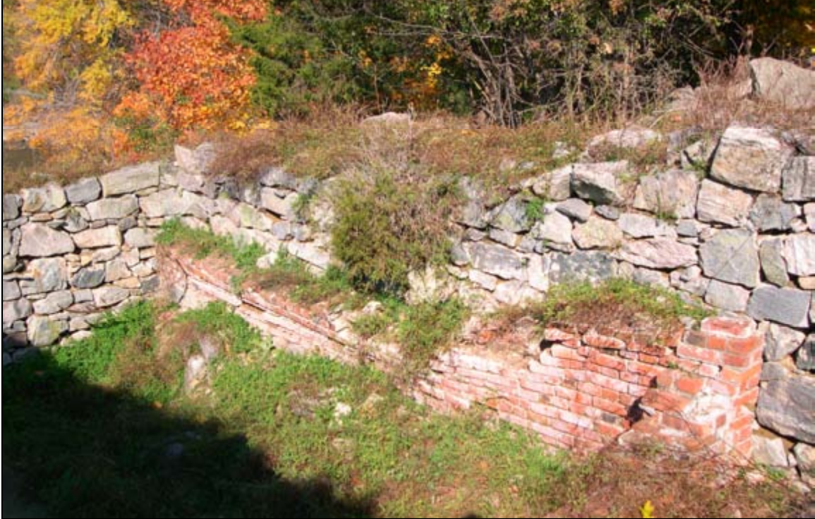
Photograph 33: Imminent Failure of Interior Brick Wall, Interior of Romans' Powder Magazine, Looking Northeast. (D. R. Cubbison, 31 October 2003)
