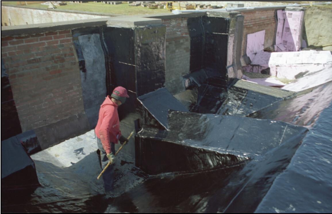
Photograph 48: View looking at the waterproofing of the casemates in Fort Macon, North Carolina. Engineers placed new lead sheeting over the old lead sheeting, and then sealed it with five coats of tar and tarpaper. A PVC drainage system was then added above the tar. (Photograph courtesy of Fort Macon State Park, Division of North Carolina Parks and Recreation.)
