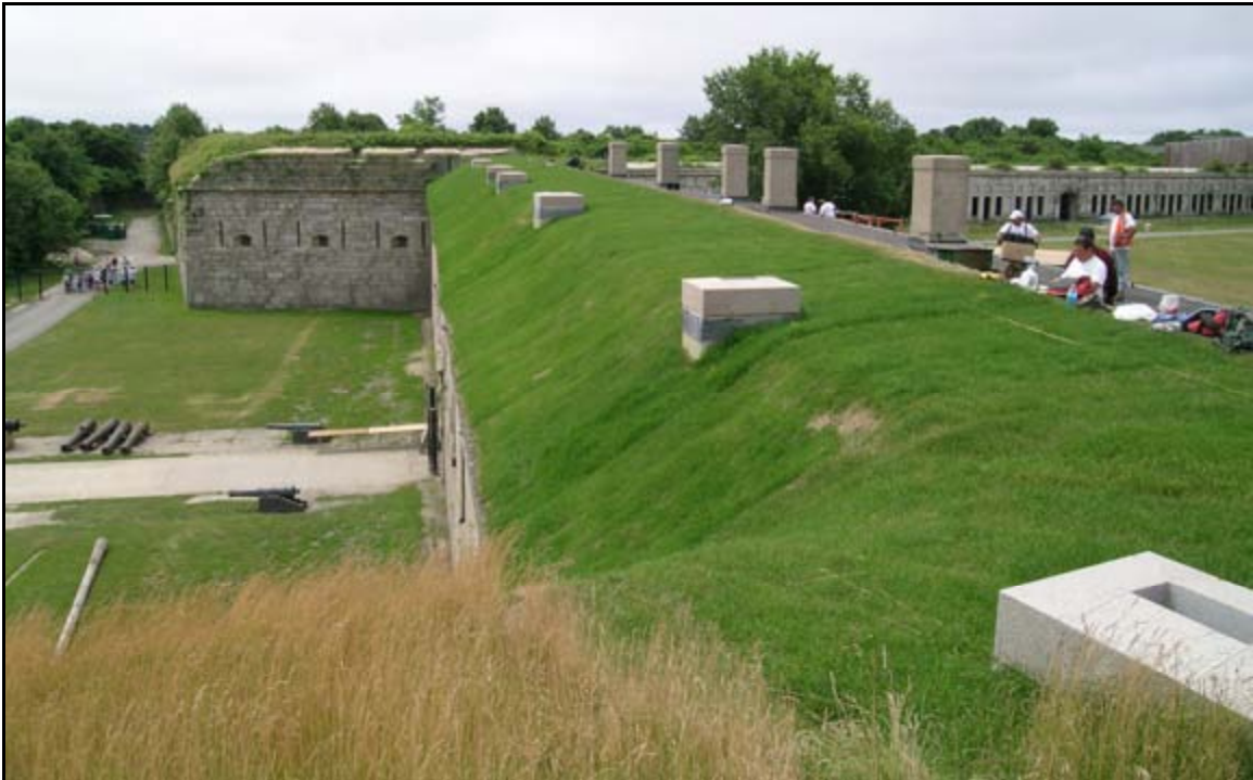
Photograph 49: View looking at earthen ramparts at Fort Adams, Newport, Rhode Island. The waterproof membrane is located underneath the earth. Workers are installing a conventional tarred roof system at the terreplein. Note the historic masonry smoke vents in the foreground.
