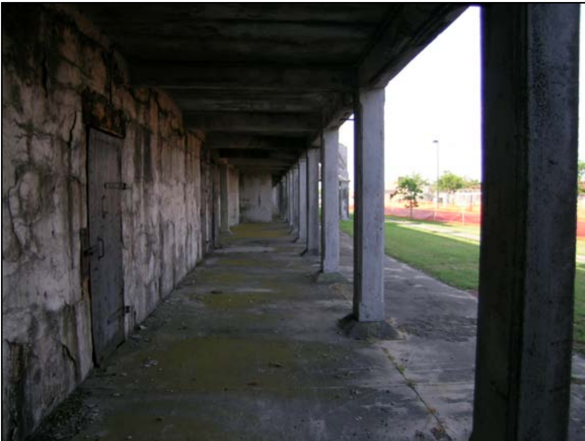
Photograph 13: View looking at the exterior of Battery DeRussy, Fort Monroe, Virginia. The doors in the left portion of this photograph prevent adequate air exchange within the battery. These doors should be opened and replaced with grates that will allow air to flow through the battery, while still preventing people from accessing the interior.
