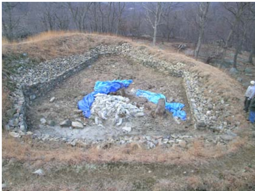
Interior of Redoubt No. 2 following demonstration project. Note stone used as "French Drains" around dry-laid stone wall. [D. Cubbison, February 2006]
