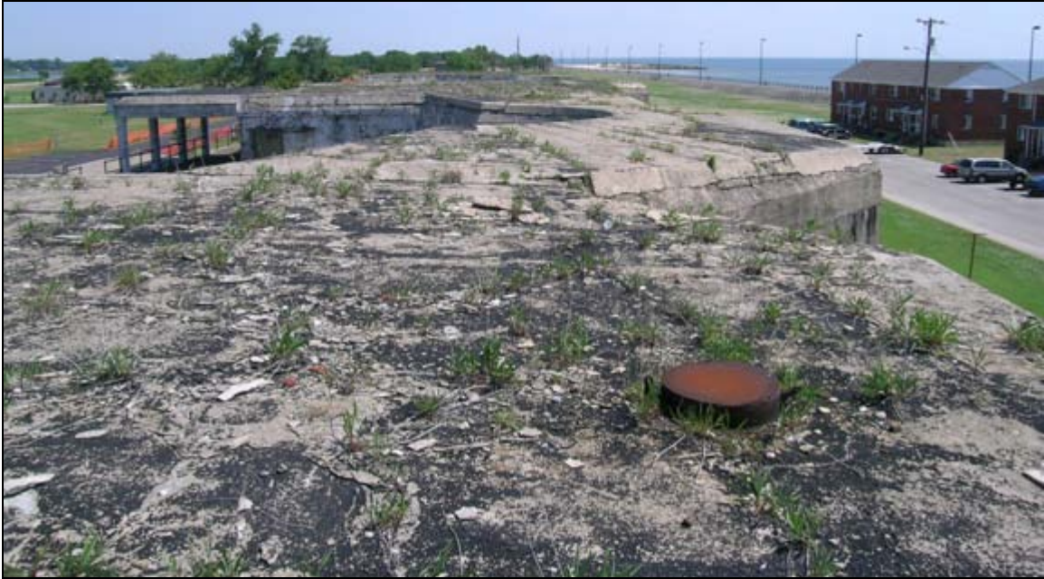
Photograph 15: View looking at the roof of Battery DeRussy, Fort Monroe, Virginia. Note how this portion of the roof has deteriorated significantly. Differences in the rate of expansion between the surface layer and the substrate cause the surface layer to disintegrate and become unattached from the substrate. Over time, this allows moisture to pool atop the fortification, exacerbating the problem.
