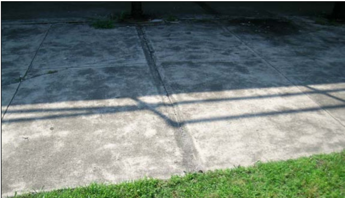
Photograph 53: View looking at the groove that leads water away from the base of the foundation at Battery DeRussy, Fort Monroe, Virginia. The slope of the earth at the junction of the concrete foundation has been raised, and water can no longer drain away from the fortification. These slopes should be re-graded to ensure that moisture flows away from the battery.
