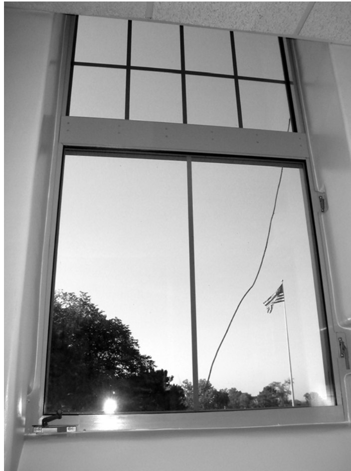
Figure 4.4. Awkward resolution of casement hardware in former double-hung window opening (Army 2004).
