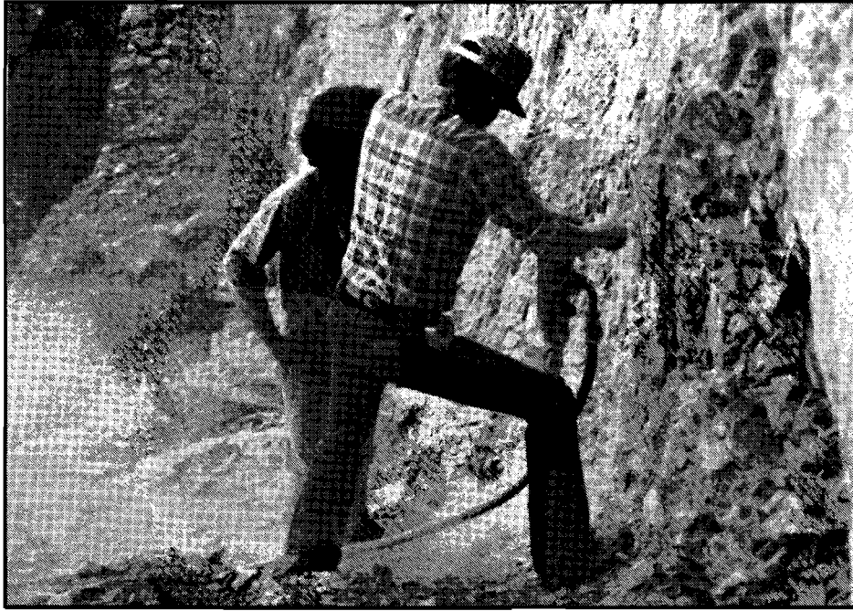
Figure P.6. George Jones and Cathy Black of Morrison-Knudsen Corporation drilling post holes for fence at AZ EE:11:30, April 1991.
