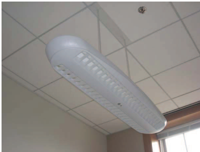
Figure 69: Private office light fixture off in an occupied office during the day
