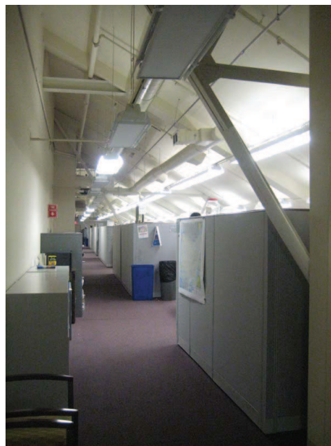
Figure 62: Previous lighting fixtures provided poor ambient lighting and did not take advantage of reflective surfaces to distribute light more evenly
