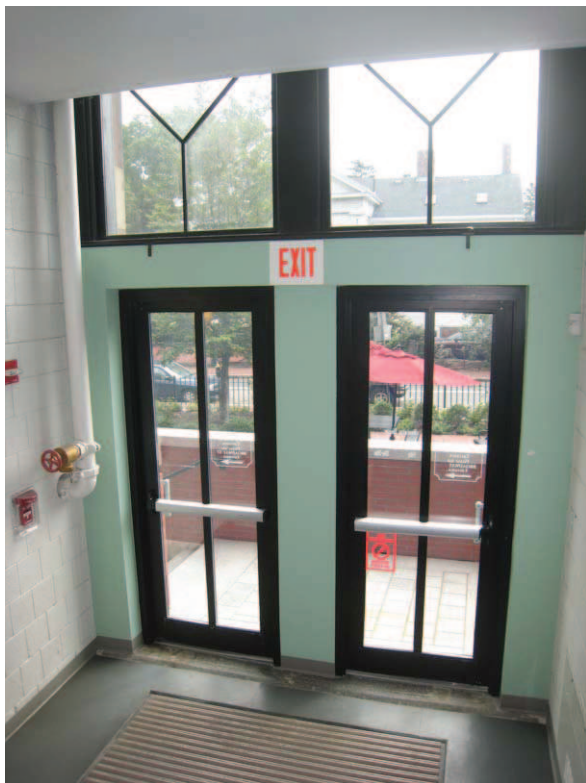
Figure 110: Views of windows from the new emergency stairwell that was added at the the Annex. The stair was held back to minimize impact on windows and to allow more daylight to penetrate the space
