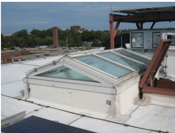
Figure 106: Roof skylights were added in 1899 and a third was added during this renovation
