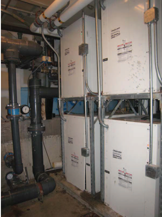
Figure 82: Power unit for ground source heat pump.
