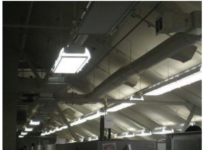
Figure 65: Fixtures added after sustainable renovation. Located in same space at opposite end of building
