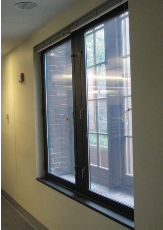
Figure 70: Note historic wood window on exterior with anodized aluminum window unit in furred-out interior
