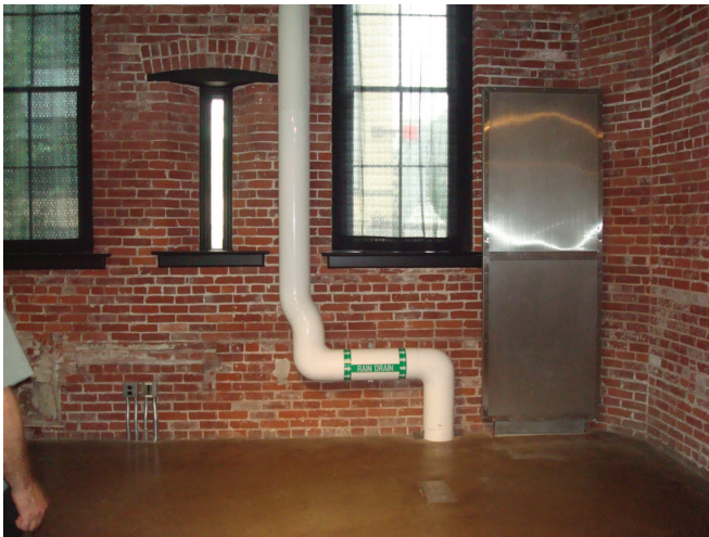
Figure 95: Pipe showing rain drain capture and flow to underground cistern
