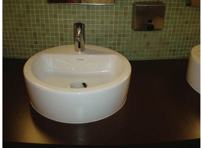
Figure 92: Sensor activated faucet at lavatory
