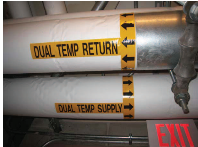
Figure 80: Ground source heat plumbing supply and return
