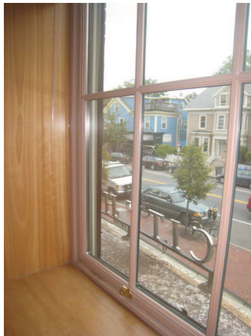
Figure 78: Close-up of window corner
