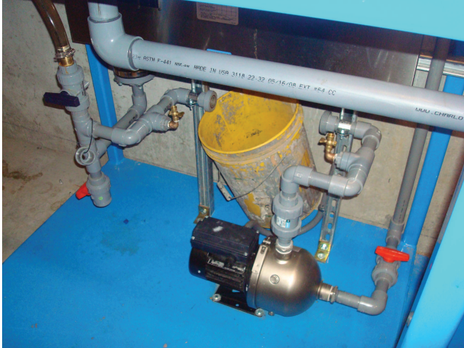
Figure 94: Pump and piping for water reuse from underground cistern
