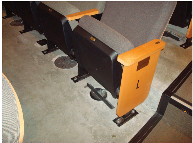
Figure 84: Each seat includes diffusers for underfloor air distribution system
