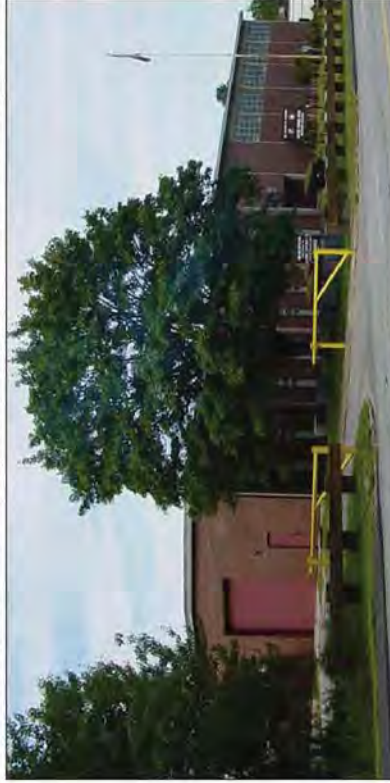
Rear of the Auburn, ME USARC. Note overhead rolling door and roof form.
