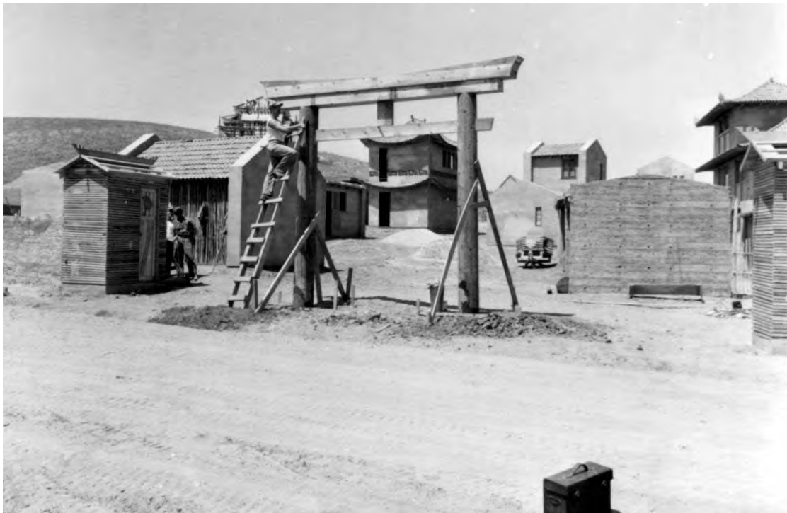
Figure 20. A shot showing construction work and buildings of combat town at Camp Pendleton, CA, 15 August 1952 (NARA College Park, RG 127-GC, box 11, photo A176772).
