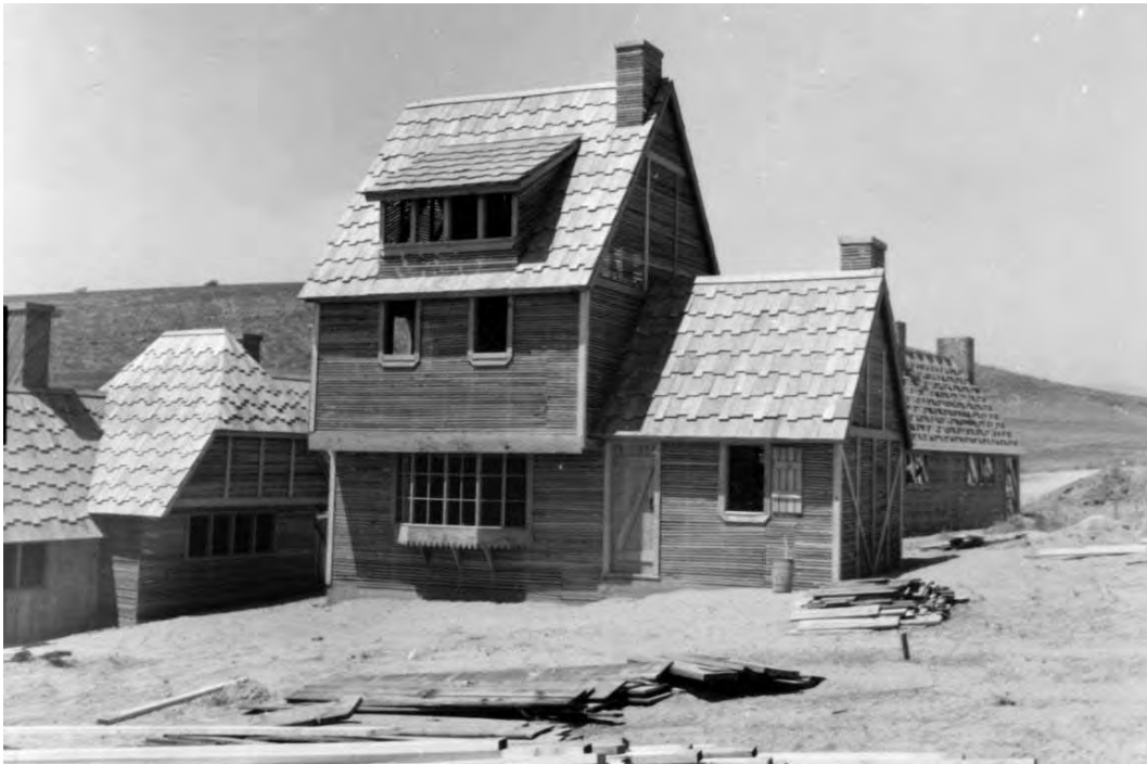
Figure 10. A building in the last stages of construction in the European section of combat town at Camp Pendleton, CA, 15 August 1952 (NARA College Park, RG 127-GC, box 11, photo A176775).
