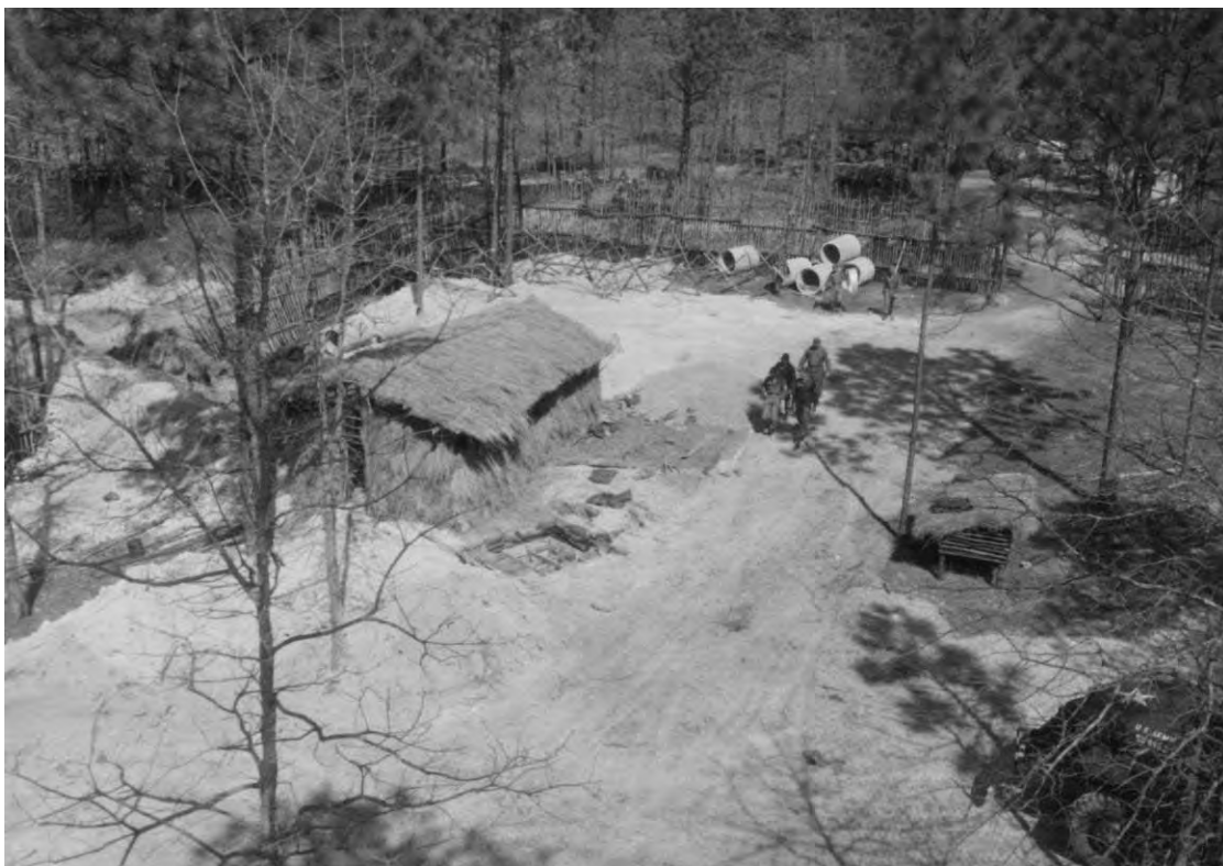
Figure 29. Construction site of Vietnamese village in "H" area at Fort Bragg, NC, 8 April 1966 (NARA College Park, RG 111-SC post-1955, photo SC628897).
