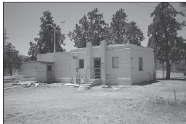
Figure 3. Building 90322 on post, formerly part of a water treatment plant, is being renovated to serve as a curation facility.
