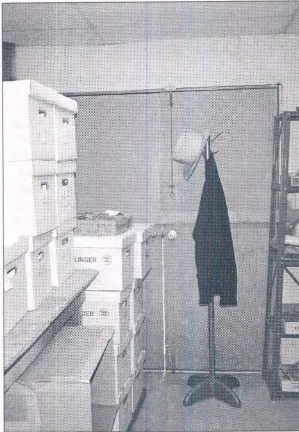
Figure 11. Exterior doors in the collections storage area. Environment and security are compromised by the gap between the doors.
