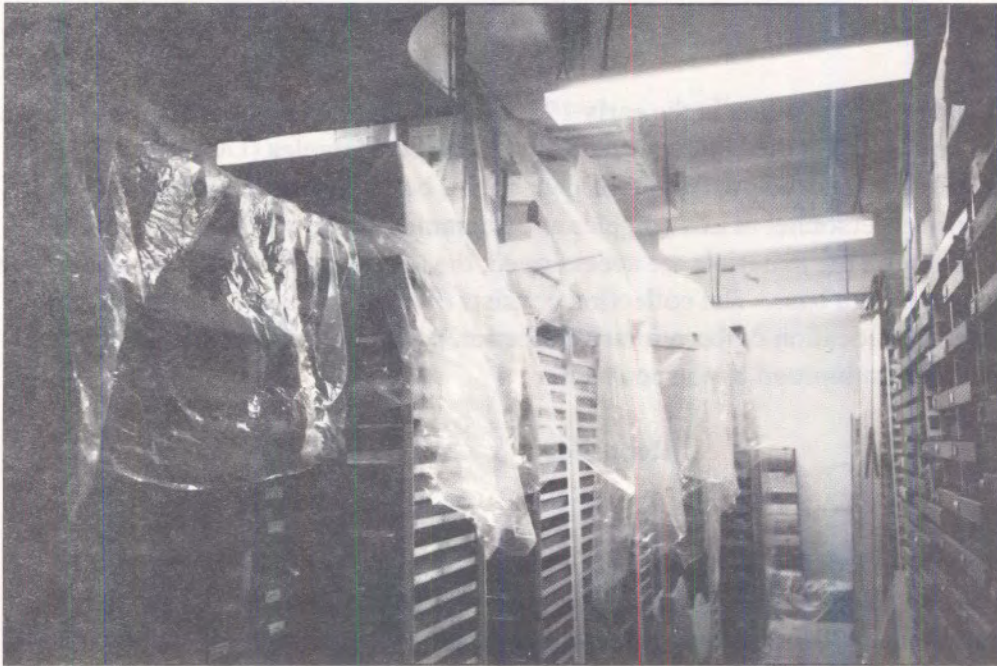
Figure 38. Interior of the repository at UCLA showing the steps that have been taken to combat the water problems.
