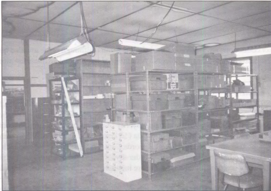
Figure 14. Collections storage at Fort Sill (note water stains on ceiling).
