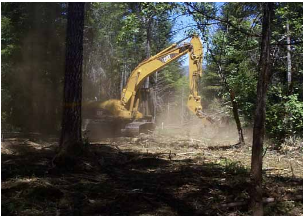
Excavator with mastication head reduces fuels within the WUI on the Medford BLM District near Grants Pass, Oregon. Credit: Bradley Washa, BLM
