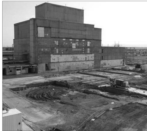
The River and Plateau Committee tracked K Basin cleanup progress in 2008, including K East Basin demolition (shown above).
