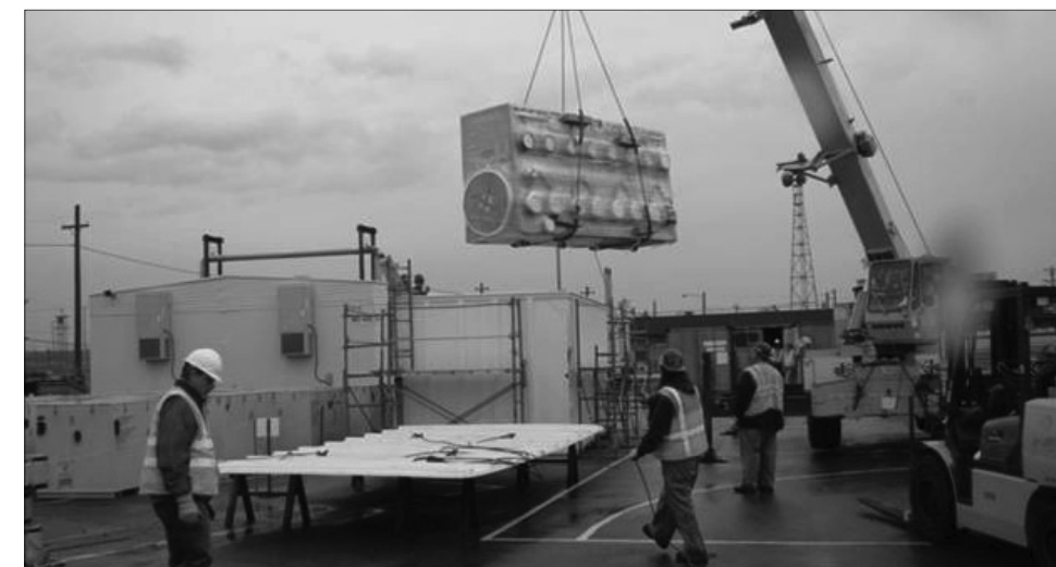
Workers load a glovebox into a waste container for eventual shipment to the Environmental Restoration Disposal Facility (ERDF).
