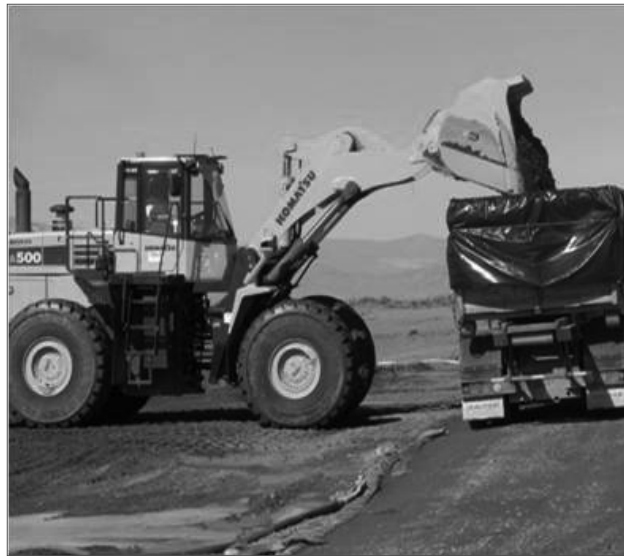
Work at the BC controlled area included soil shipments to ERDF. In October, the area was seeded with a mix of predominantly native grass species as an interim soil stabilizer prior to full revegetation.
