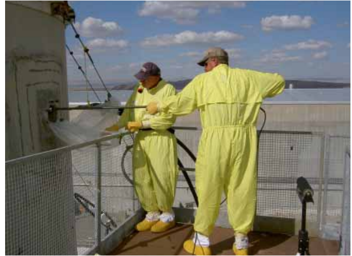
Workers work on the PUREX stack probe replacement that serves the PUREX plant.
