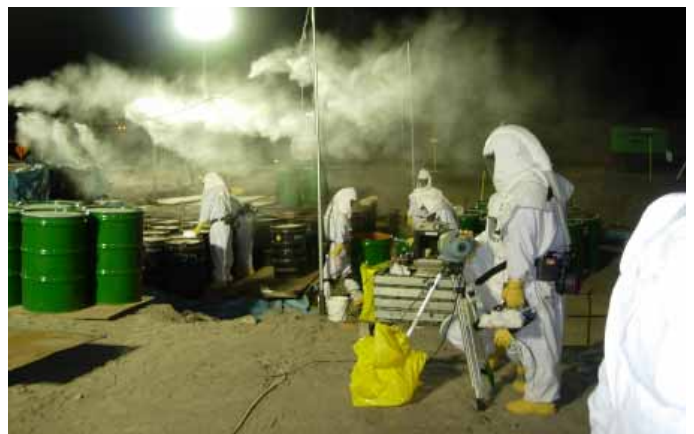
Workers use an open-air misting system to control contamination during waste retrieval.
