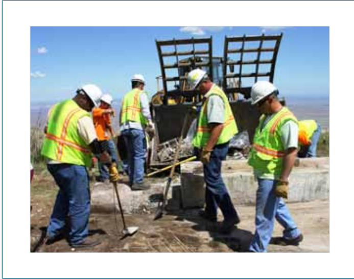
Workers clean up the former site of the 6652-T Fire Protection Lower Pump House on the upper Arid Lands Ecology Reserve.
