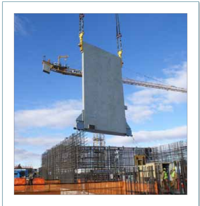
An 85-ton shield door built for the WTP Pretreatment Facility is transported for installation.
