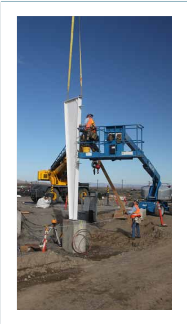
Workers secure a section of structural steel for the Radiological Treatment Building of the 200 West Groundwater Treatment System.
