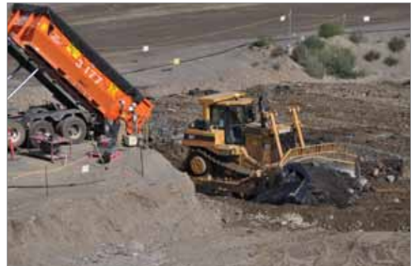
A load of waste is spread out by bulldozer at the bottom of the 70-foot-deep Environmental Restoration Disposal Facility.
