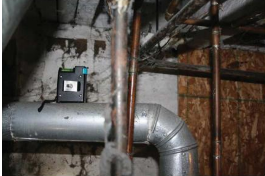
Inspection #59: The vent on the hot water heater has a negative slope, which prohibits gases from venting properly. The Authority did not identify this violation during its February 3, 2012, inspection.
