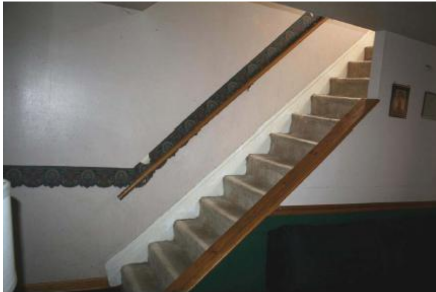
Inspection #55: The stairway on the first floor requires a guardrail on the open side. The Authority did not identify this violation during its February 16, 2012, inspection.
