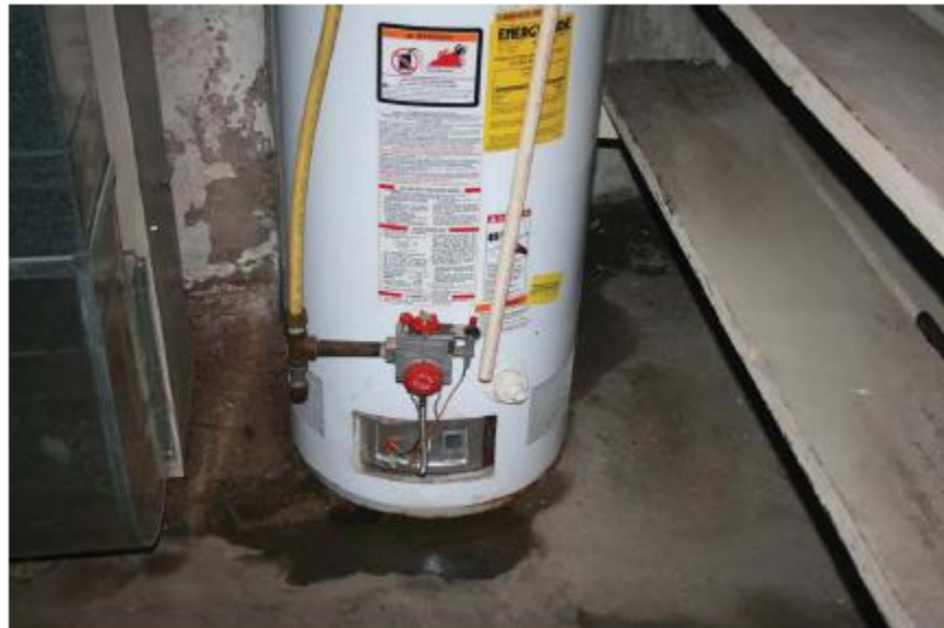
Inspection #62: The pressure relief valve discharge tube is more than the required 6-inch maximum distance from the floor. The Authority did not identify this violation during its March 1, 2012, inspection.
