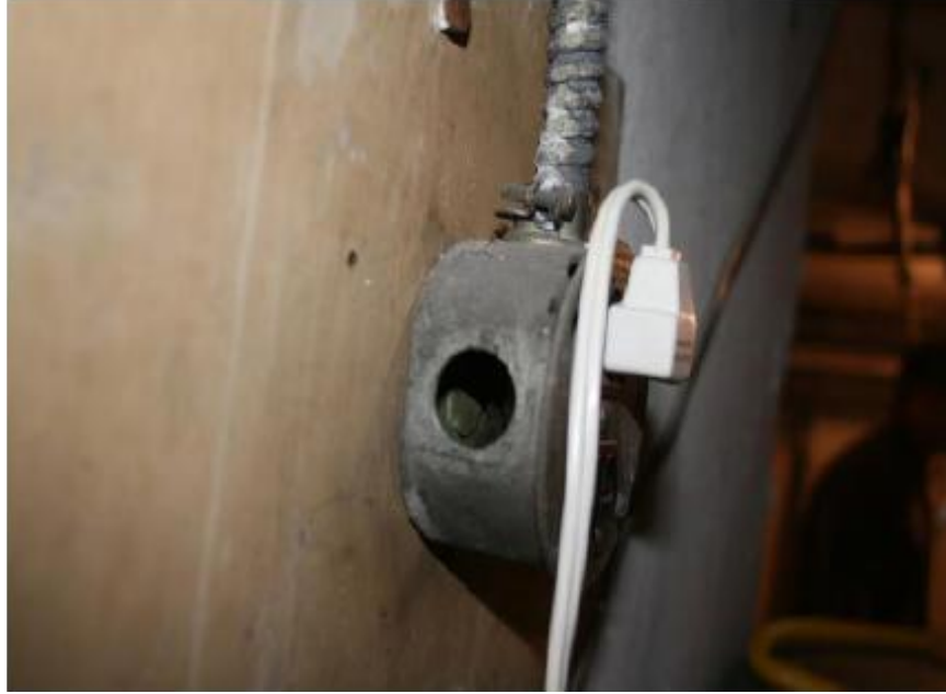
Inspection #52: The junction box above the washing machine is missing a knockout plug creating a potential shocking hazard. The Authority did not identify this violation during its February 1, 2012, inspection.
