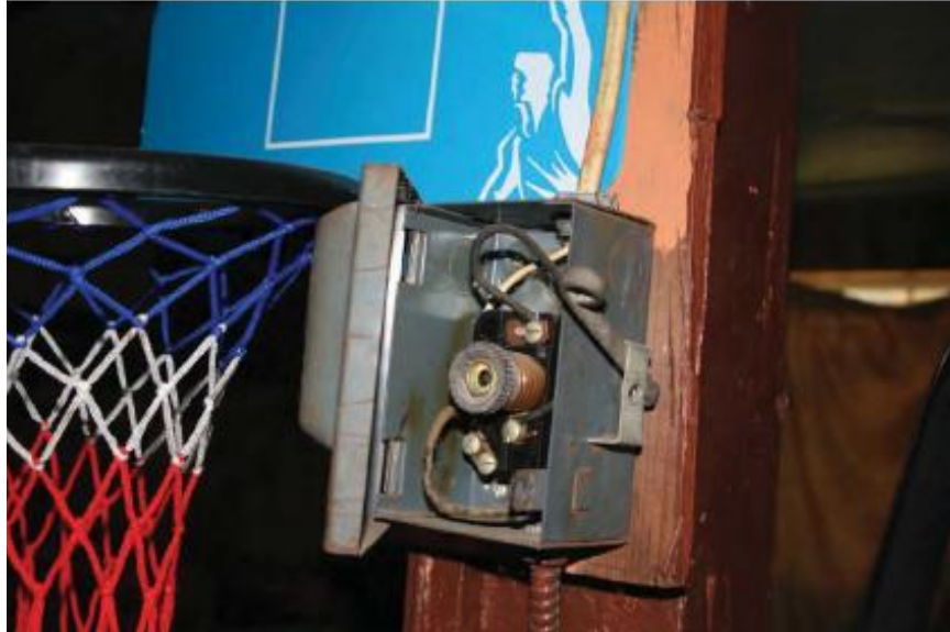
Inspection #3: The basement fuse box is not secure and contains exposed wires and contacts. The Authority did not identify this violation during its February 29, 2012, inspection.
