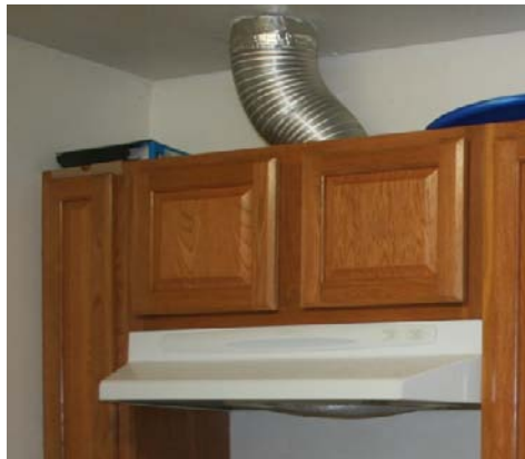
Improper sealing material used to connect tubing to ceiling
