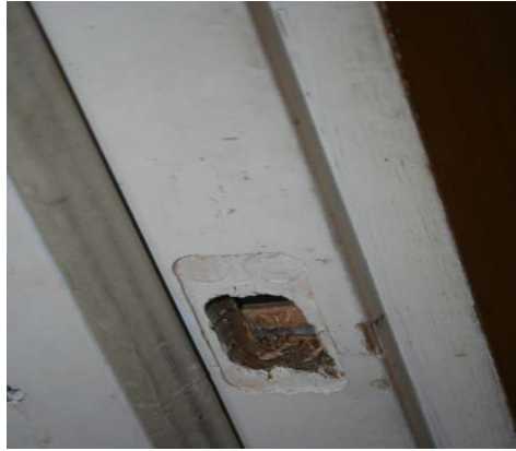
Missing door striker to rear entrance
