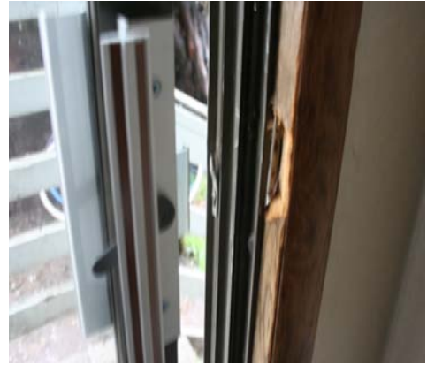
Missing door striker to rear entrance of bedroom
