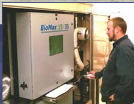
Automatic Control System
