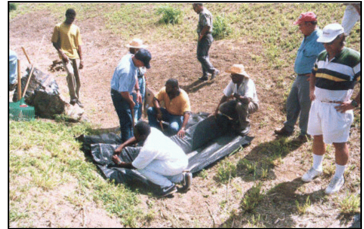
Figure 23. Erosion & Sediment Control Workshop trainees install a Triangular Silt Dike™ check dam in Estate St. George's Hill, St. Croix, June 1998.
