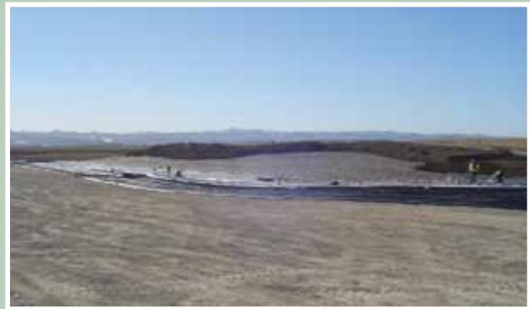
MINS installed the IA-H1 landfill cap over the Containment Area covering approximately 73 acres of the IA-H1 site. The gentle sloping of the cap design decreases potential erosion and thus decreases maintenance costs. In this photo, the field team is installing the geo-composite venting layer.
