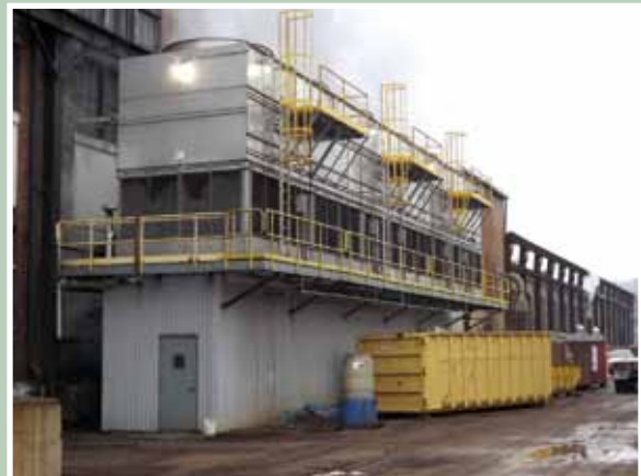
The Production Shop covers approximately 4.5 acres. Rain water is collected from approximately 2.2 acres of this roof. On average, the system collects and stores more than 2.5 million gallons of rainwater each year as cooling water for the plant's production operations.
