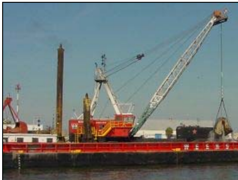
Figure 4-2 Conventional Spudded Leg Clamshell Dredge (courtesy of U.S. Army Corps of Engineers)
