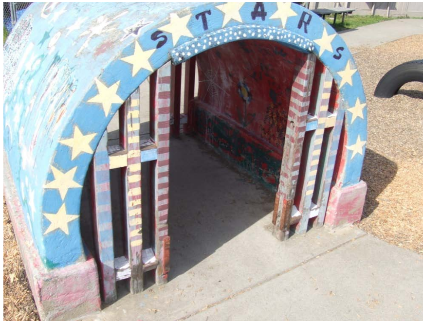
Photograph 20 – Taken at Fort Bragg on 4/1/10 showing peeling paint on the wooden portion of a concrete play tunnel on the playground.
