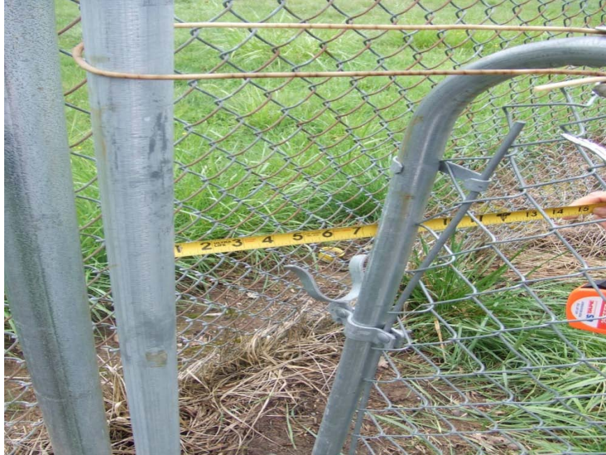
Photograph 7 – Taken at Willits Head Start on 4/1/10 showing an improperly secured gate that led from the playground to an unsupervised area. The gate latch was within children’s reach.
