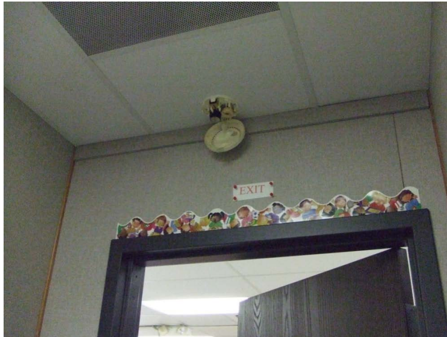
Photograph 18 – Taken at Fort Bragg on 4/1/10 showing a nonfunctioning smoke detector in the hallway.
