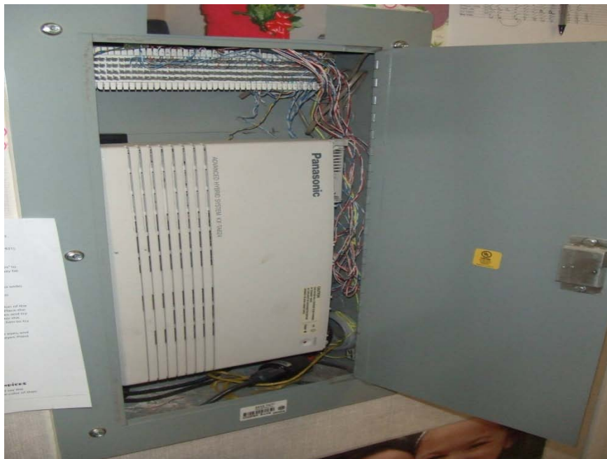
Photograph 24 – Taken at Low Gap on 4/2/10 showing the central telephone wiring system in an unlocked wall-mounted case within children’s reach.
