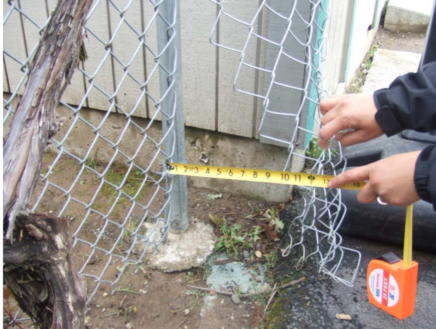
Photograph 11 – Taken at Willits Head Start on 4/1/10 showing a chain-link fence on one part of the playground that was not properly fastened to the fencepost, creating a 10-inch gap that led to the water-filled hole and the unsupervised field shown in Photographs 9 and 10.
