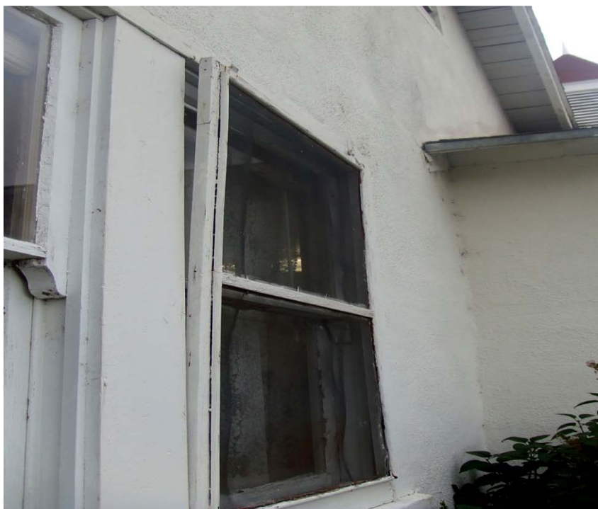
Photograph 6 – Taken at Lone Pine on 6/3/09 showing a broken window screen.
