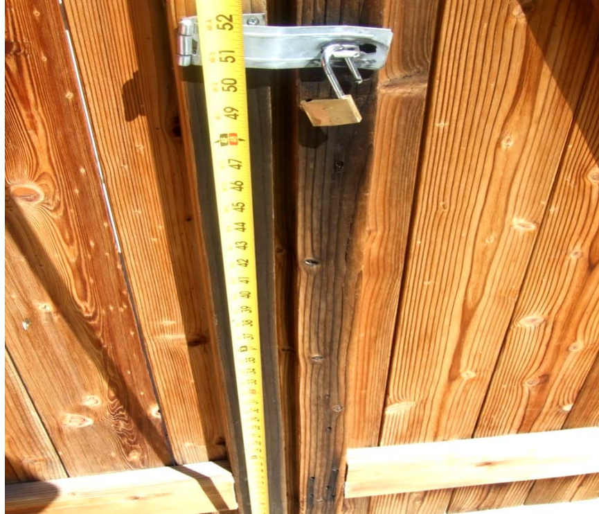
Photograph 9 – Taken at Lee Vining on 6/4/09 showing an unlocked playground gate that led to street parking. The gate was within children’s reach.
