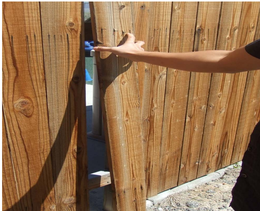
Photograph 8 – Taken at Lee Vining on 6/4/09 showing loose boards and protruding nails on the playground fence.
