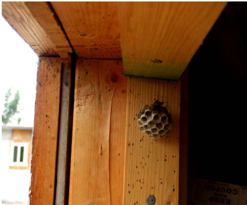
Photograph 4 – Taken at Little Promises on 6/3/09 showing a yellowjacket hive on the inside of the door of an unlocked storage shed on the playground.
