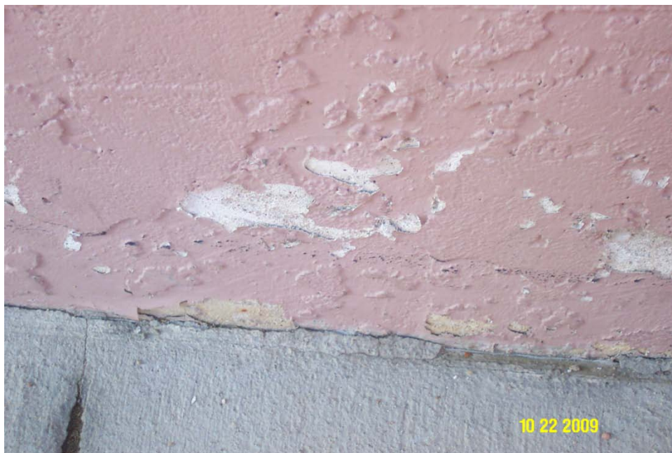
Photograph 2 – Taken at the Powell facility on 10/22/2009 showing chipped paint on a playground wall.
