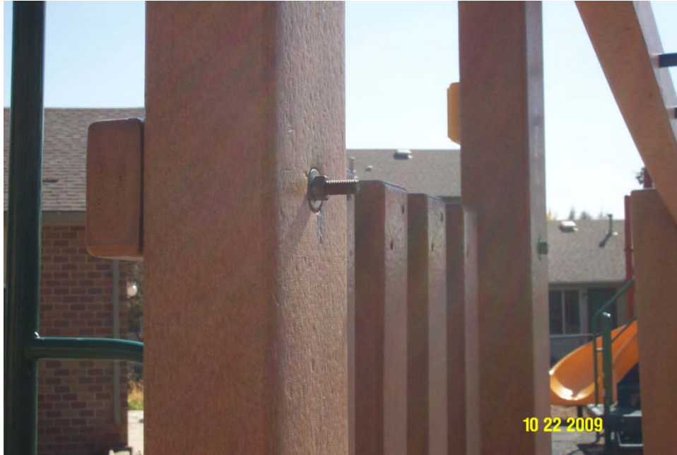
Photograph 3 – Taken at the Casa de la Esperanza facility on 10/22/2009 showing the threaded end of a bolt protruding from a piece of playground equipment at child level.
