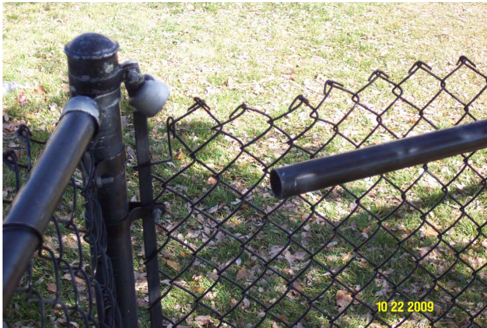
Photograph 4 – Taken at the Casa de la Esperanza facility playground on 10/22/2009 showing the top rail of the fence separated from the fencepost.
