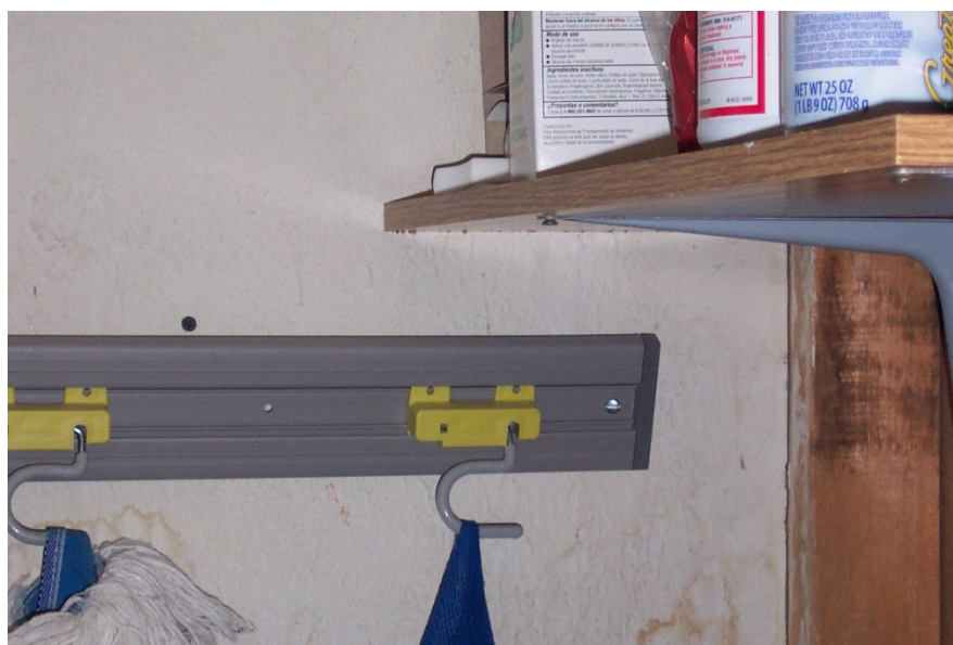
Photograph 2 – Taken at the Saguache facility on 5/20/2009 showing potentially flammable cleaning supplies next to the furnace. Together, Photographs 1 and 2 show the proximity of the cleaning supplies to the furnace; i.e., the tip of the shelf shown in Photograph 2 can also be seen in the upper-right corner of Photograph 1, and the dust mop can be seen in both photographs.
