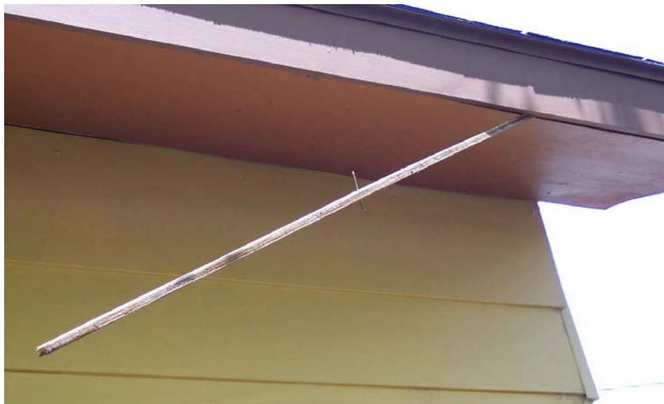
Photograph 5 – Taken at the Saguache facility on 5/20/2009 showing broken trim with a protruding nail above the playground area.
