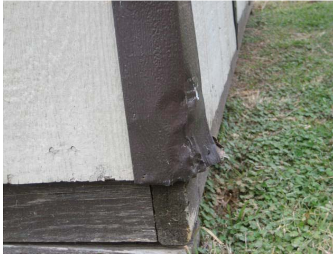
Photograph 1 – Taken at Archer City on 1/13/10 showing a playground storage shed with a strip of sheet metal having sharp, jagged edges.
