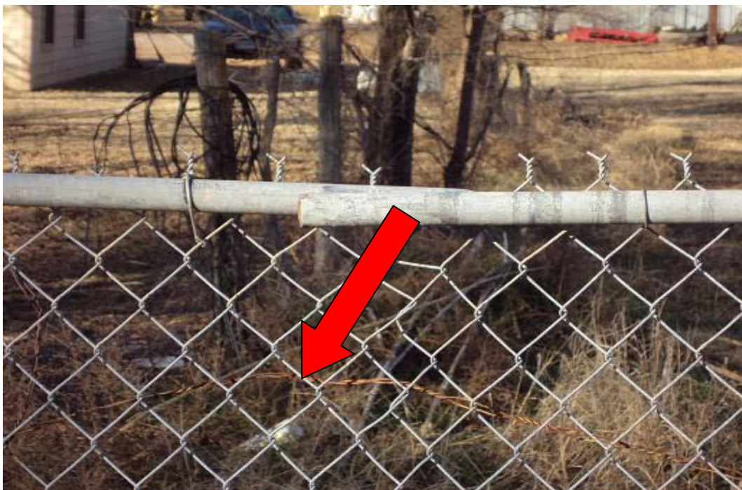
Photograph 9 – Taken at Dunbar on 1/12/10 showing barbed wire running through the playground fence and sharp, twisted chain-link ends at the top.
