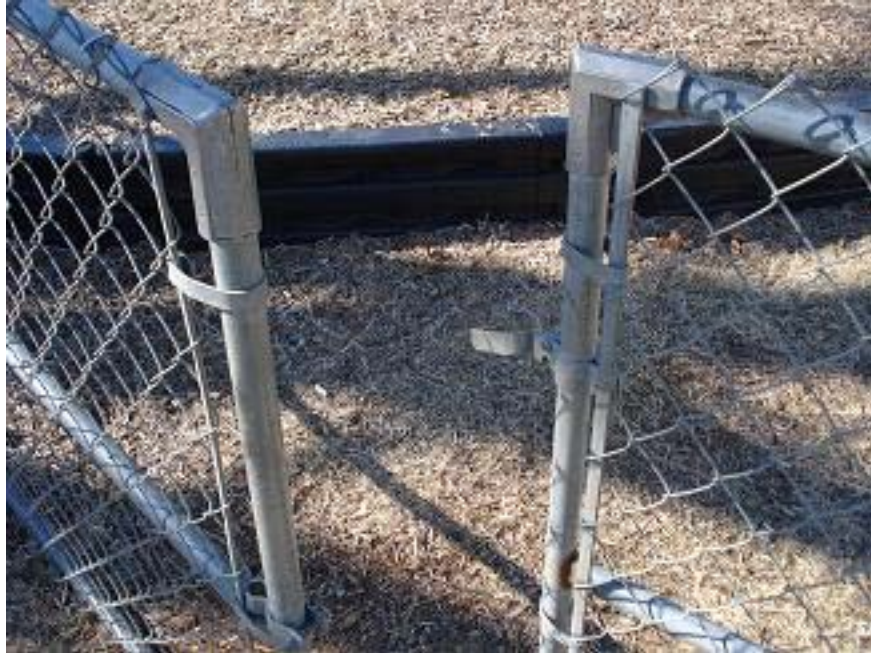
Photograph 3 – Taken at Chillicothe on 1/13/10 showing a playground gate that could not be secured because of a gap between the latch and the post. The gate opened to the facility’s parking lot.
