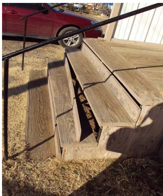
Photograph 10 – Taken at Dunbar on 1/12/10 showing loose boards on steps to the facility's main entrance.
