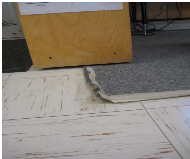
Photograph 6 – Taken at Graham on 1/11/10 showing a rug with curled edges, creating a tripping hazard.
