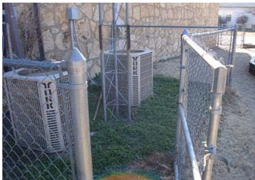
Photograph 13 – Taken at Turner on 1/12/10 showing an unlocked playground gate leading to a radio tower and two air conditioning units.
