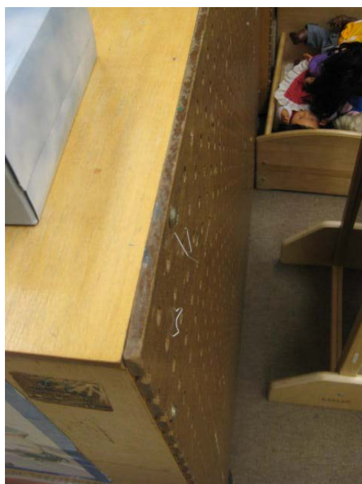
Photograph 14 – Taken at Seymour on 1/13/10 showing the sharp ends of staples protruding from a bookcase in a classroom.
