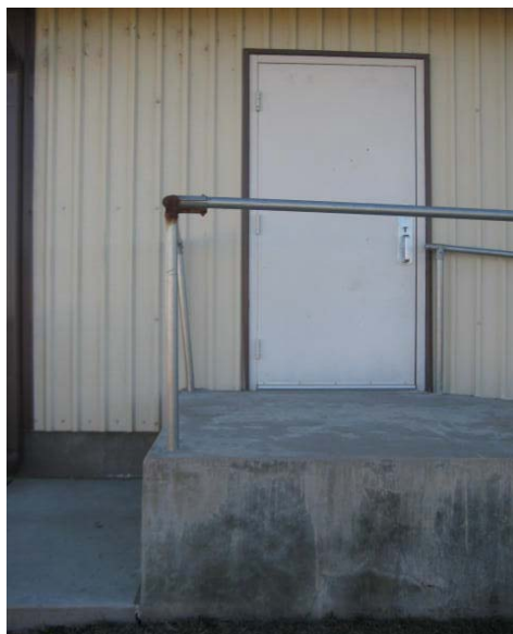
Photograph 8 – Taken at Olney on 1/11/10 showing a platform more than 20 inches high without sufficient protective barriers.
