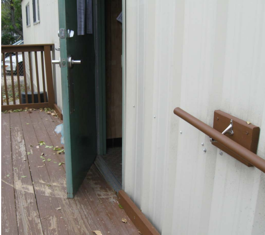
Photograph 5 – Taken at Comal No. 1 on 12/16/09 showing a portable classroom building door that was difficult to open. Opening the door beyond this point required significant effort because the door scraped the deck.
