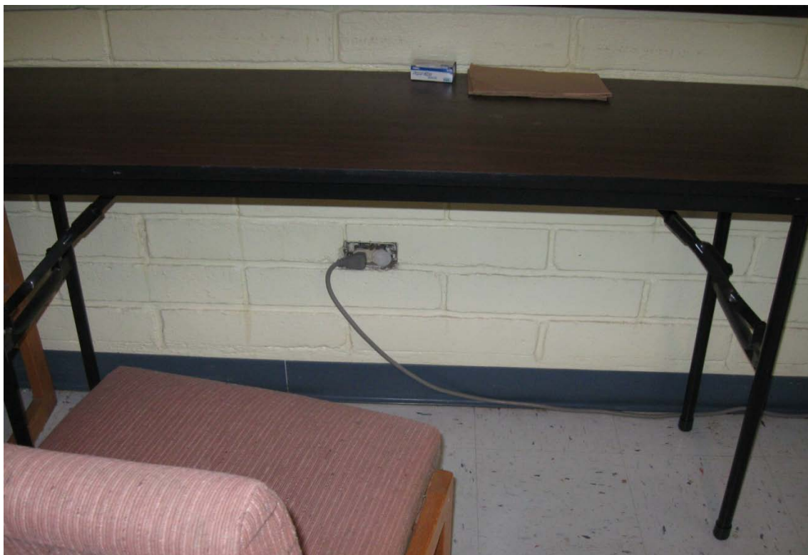
Photograph 2a – Taken at Comal No. 1 on 12/16/09 showing an outlet in a main hallway that lacked a wallplate. The wires in the wall were accessible.
