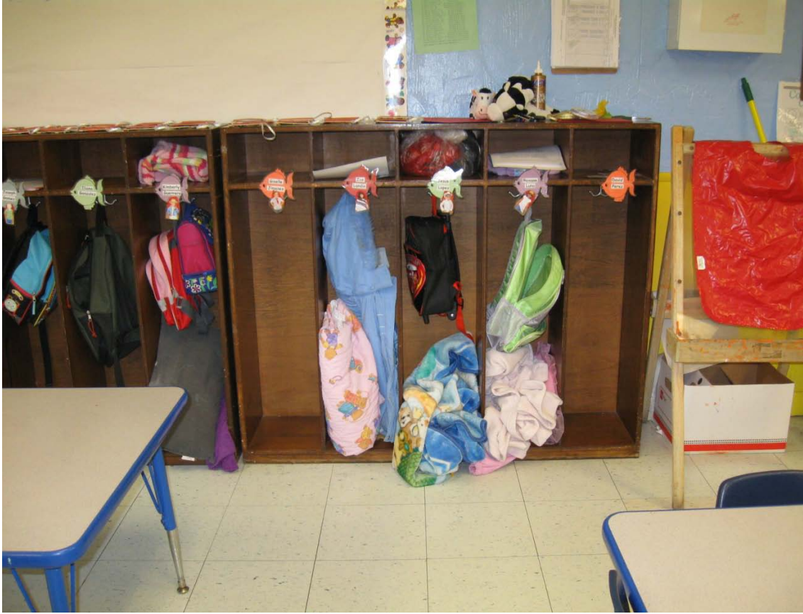
Photograph 8 – Taken at Comal No. 4 on 12/16/09 showing lockers that were not attached to the wall. We witnessed one set of lockers pulling away from the wall as a child pulled her coat from a hook at the top of a locker.
