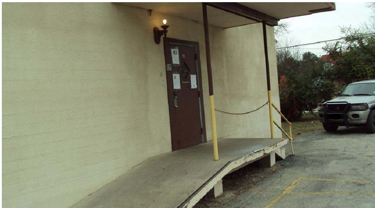
Photograph 10 – Taken at Seguin on 12/16/09 showing an unlocked side door that allowed unrestricted access to the building. The door opened to a hallway where classrooms were located.
