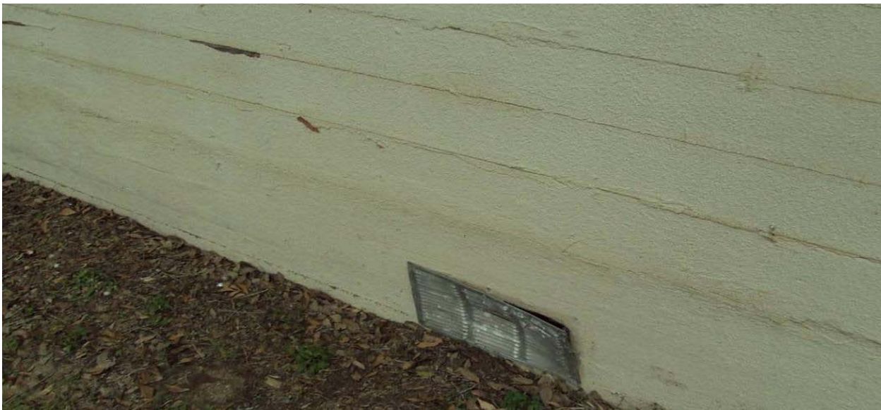
Photograph 9 – Taken at Seguin on 12/16/09 showing a partly detached vent cover with sharp edges at the bottom of an exterior wall.
