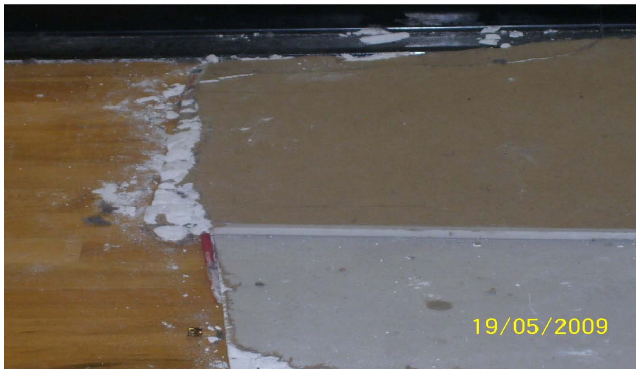
Photograph 3 – Taken at Sixth Street on 5/19/09 showing broken drywall and debris on the floor of a gymnasium where children routinely played.
