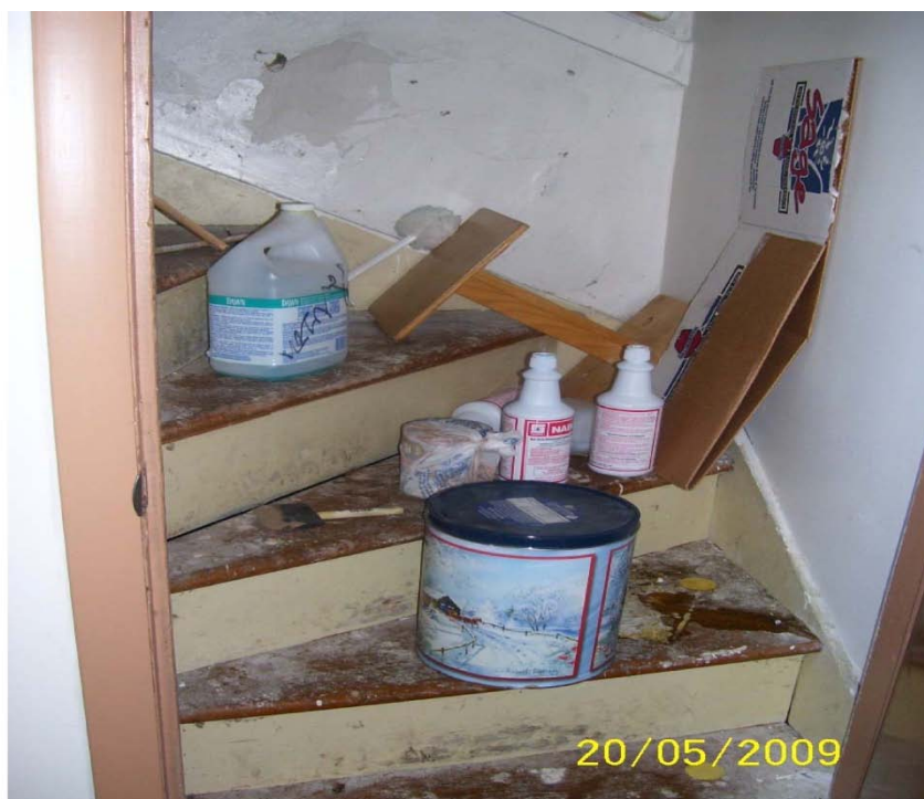
Photograph 6 – Taken at Lisbon Avenue on 5/20/09 showing paint and cleaning supplies in an unlocked stairwell.
