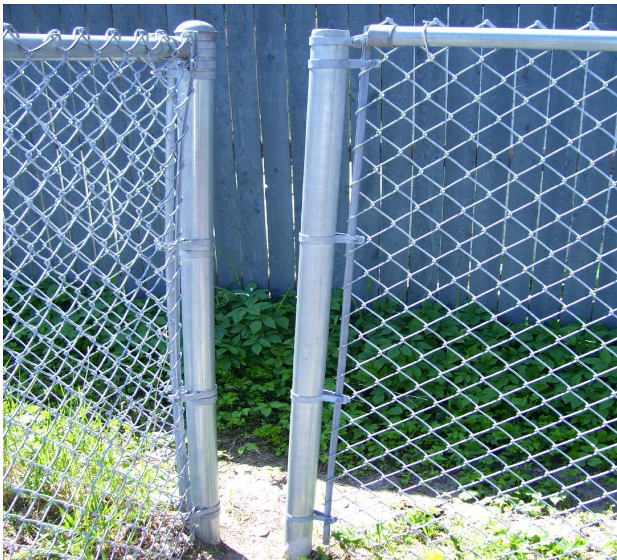
Photograph 7 – Taken at Fond du Lac Avenue on 5/20/09 showing an approximately 6-inch-wide gap in the playground fence.
