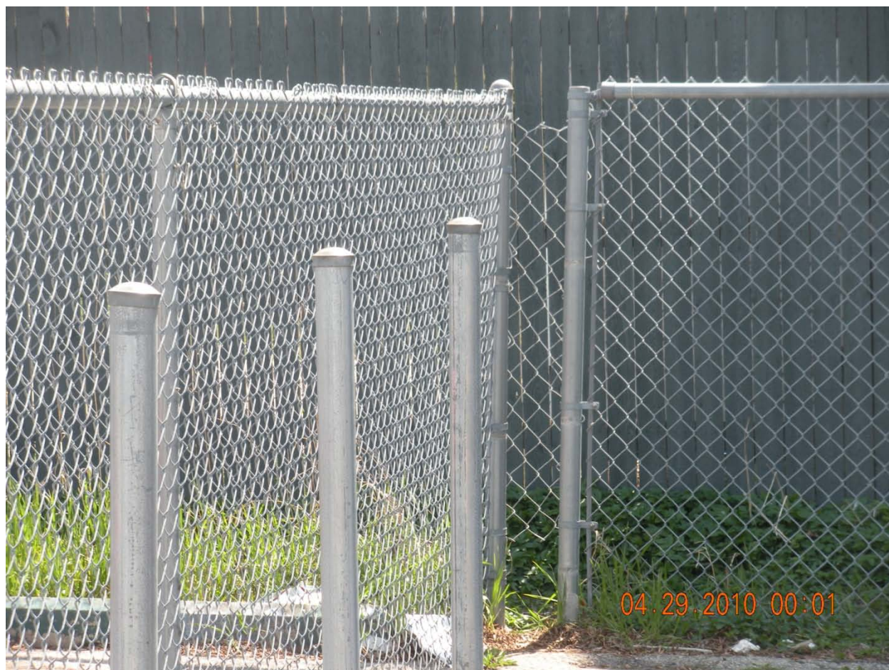
Corrected photograph 7-gap in fence enclosed
