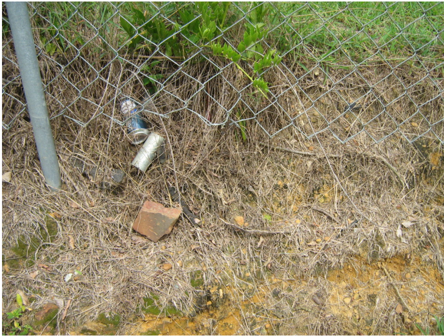
Photograph 9 – Taken at the Turner County Head Start center on 8/26/2009 showing debris around a playground fence and a gap between the fence and the ground.
