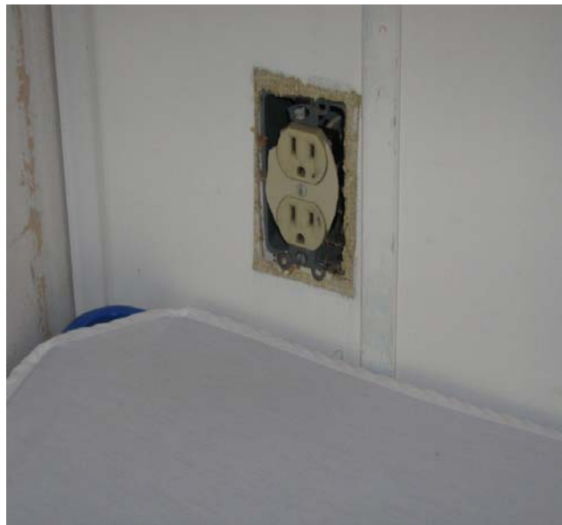
Photograph 2 – Taken at the Hahira Head Start center on 8/25/2009 showing an outlet in the children's bathroom without a faceplate or protective caps.
