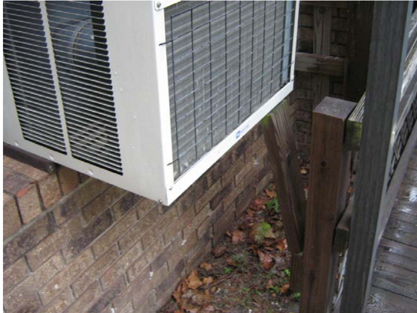
Photograph 11 – Taken at the B. W. Lester Head Start center on 8/27/2009 showing a window air conditioner partially supported by an unsecured board adjacent to the walkway to the playground.
