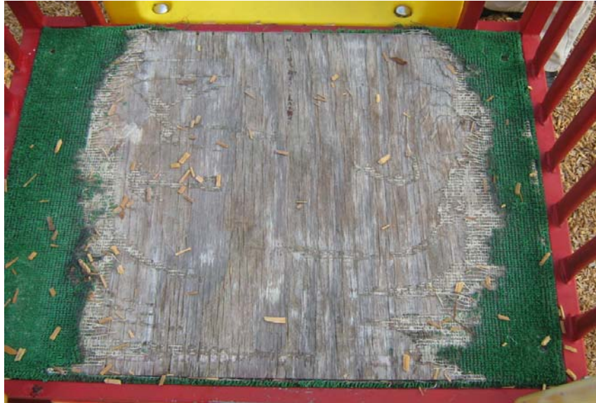
Photograph 1 – Taken at the Hahira Head Start center on 8/25/2009 showing frayed carpet covering wood at the top of a playground slide.
