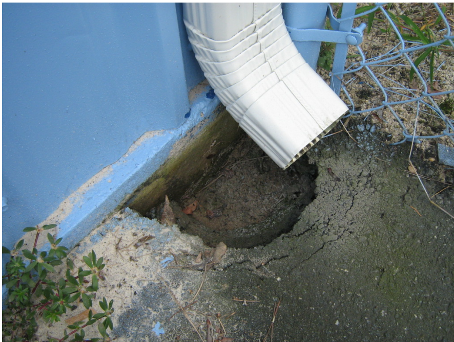
Photograph 10 – Taken at the Lowndes 1 Head Start center on 8/27/2009 showing a sinkhole in the asphalt under a gutter downspout on the playground.
