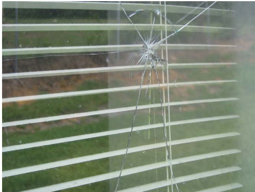
Photograph 8 – Taken at the Turner County Head Start center on 8/26/2009 showing a broken classroom window facing the playground.
