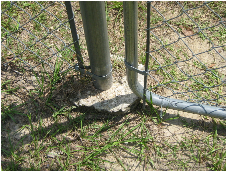
Photograph 3 – Taken at the Cook Head Start center on 8/25/2009 showing sharp edges on the concrete base of a playground fencepost.
