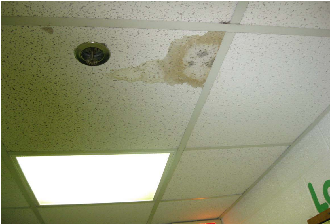
Photograph 8 – Taken at ECDC #10 on 8/17/2009 showing water-stained ceiling tiles that appeared to be moldy.
