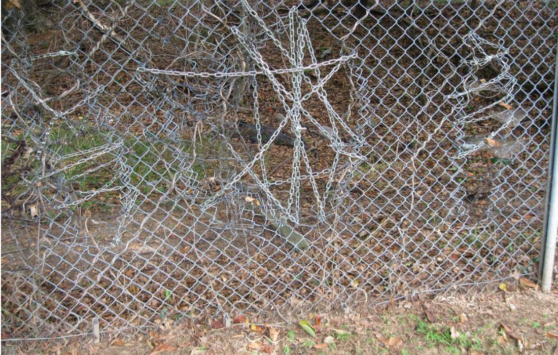
Photograph 3 – Taken at ECDC #3 on 8/20/2009 showing holes in the fence enclosing the play area that had been repaired with chains and locks. The chains and locks had sharp edges that exposed children to possible injury.
