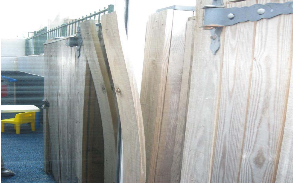
Photograph 5 – Taken at ECDC #9 on 8/18/2009 showing the wooden fence enclosing the play area. Some of the boards were loose and had protruding nails that exposed children to possible injury.
