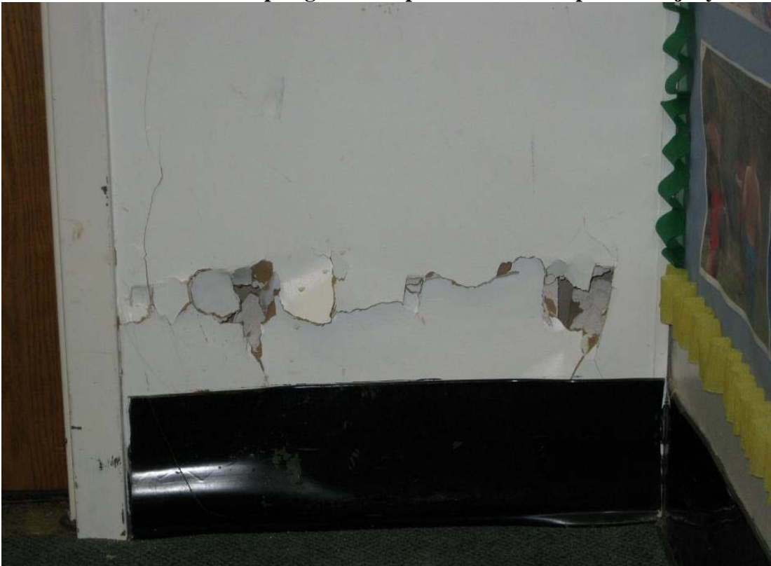
Photograph 4 – Taken at ECDC #5 on 8/11/2009 showing holes in the wall near the front door of the facility.
