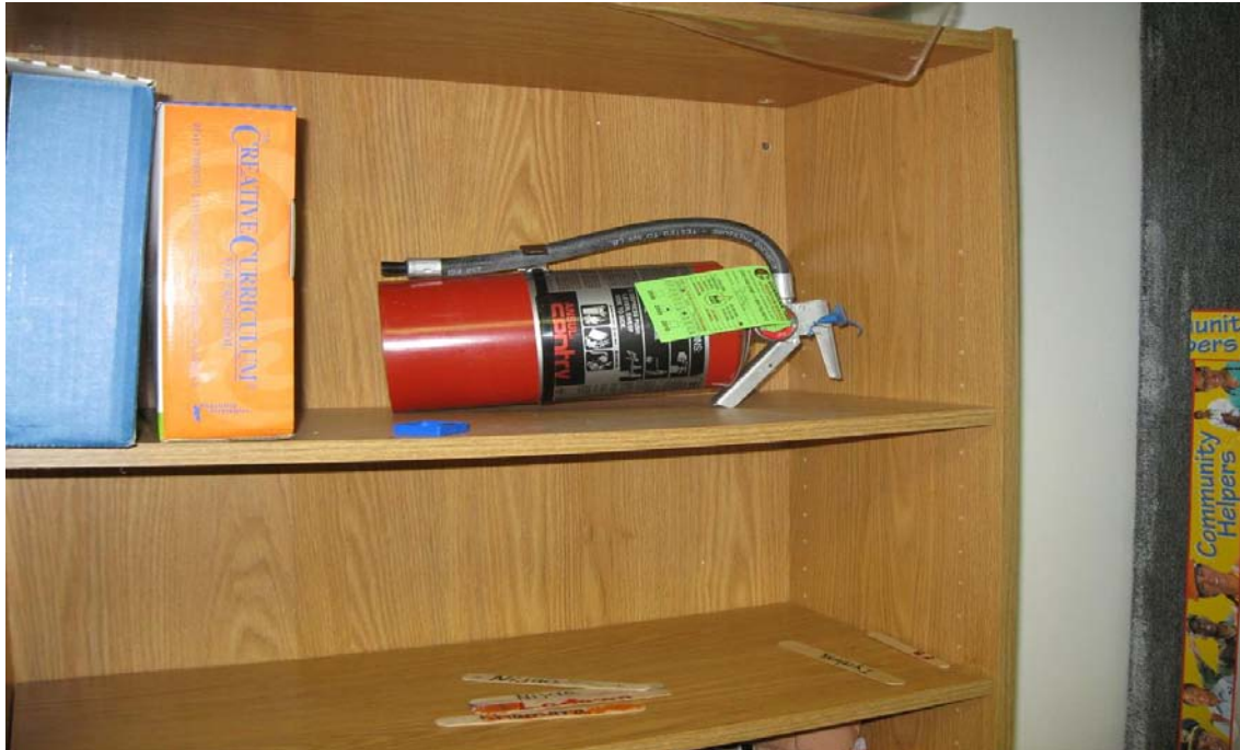
Photograph 11 – Taken at Sunshine Learning Center on 10/21/2009 showing a fire extinguisher on a shelf accessible to children.
