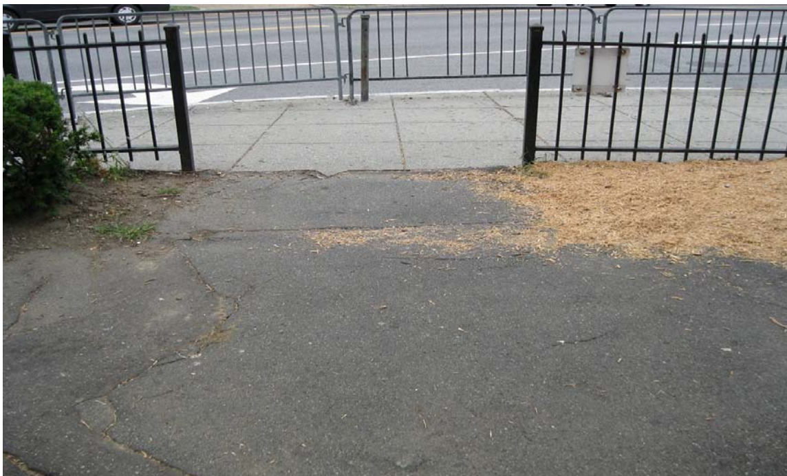
Photograph 2 – Taken at the Dance Institute on 8/11/2009 showing that the entrance to the outdoor play area did not have a gate, allowing children to leave the premises and unauthorized people to enter the play area.
