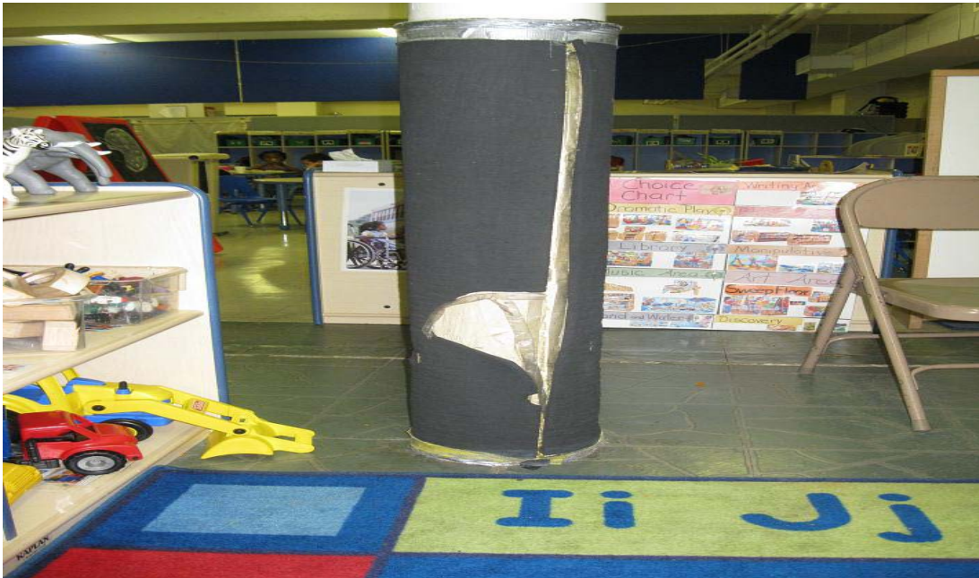
Photograph 1 – Taken at ECDC #1 on 8/12/2009 showing torn padding covering a concrete pillar in the middle of the play area, exposing children to possible harm.
