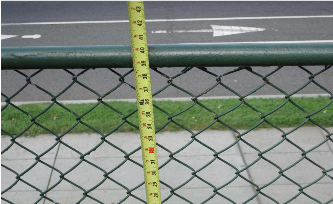
Photograph 1 – Taken at ECDC #1 on 8/13/2009 showing that the fence enclosing the outdoor play area was 40 inches high rather than the required 48 inches.
