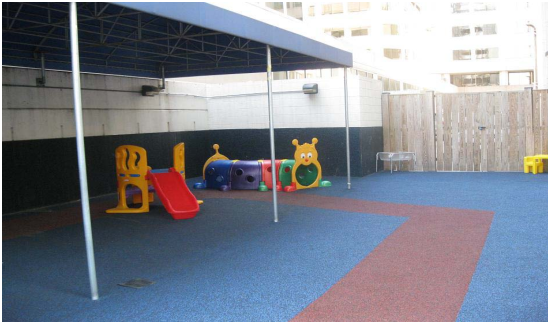
Photograph 6 – Taken at ECDC #9 on 8/18/2009 showing four metal support posts in the middle of the outdoor play area. The posts were unpadding and exposed children to possible injury.
