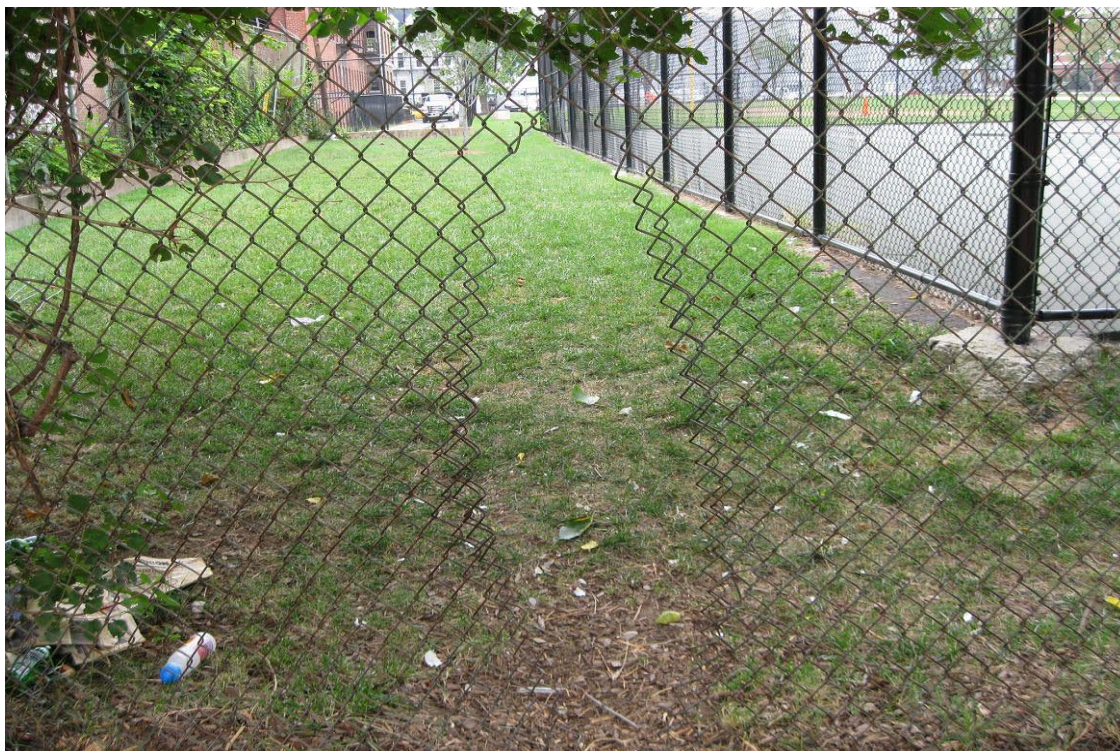
Photograph 3 – Taken at the Dance Institute on 8/11/2009 showing a hole in the fence enclosing the outdoor play area that allowed children to enter unsafe and unsupervised areas.
