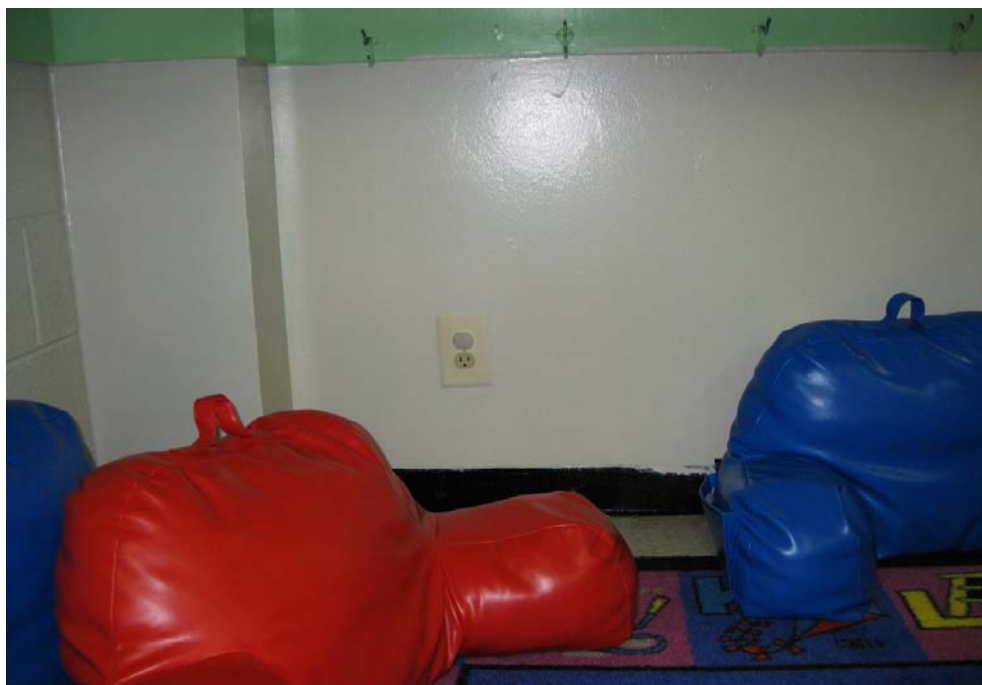
Photograph 2 – Taken at the Azeze Bates Center on 6/2/2009 showing an uncovered electrical outlet in the children's play area.
