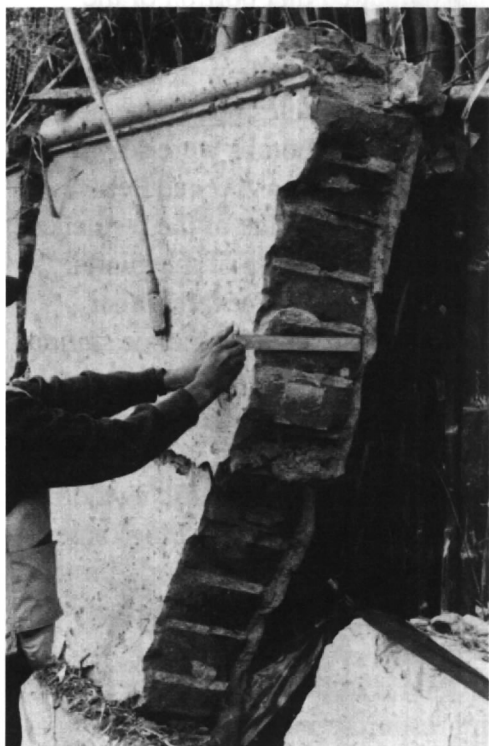
February 11, 1992—Lima, Peru: Part of the exterior wall damaged in the explosion at the U.S. Ambassador's residence.
