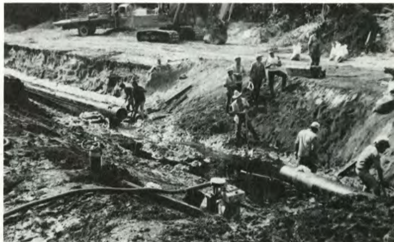
January 1–December 31, 1993: Though a few years old, these photos are indicative of the bombings currently taking place along the Cano Limon-Covenas pipeline.
