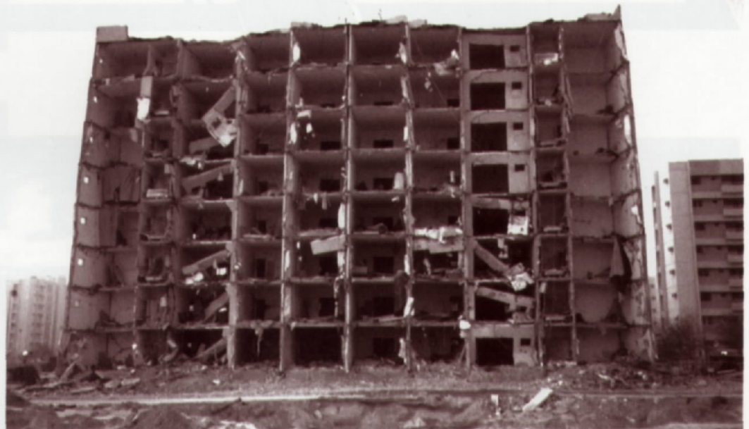
June 25, 1996—Dhahran, Saudi Arabia: Aftermath of the bombing of the al-Khobar military housing complex.
