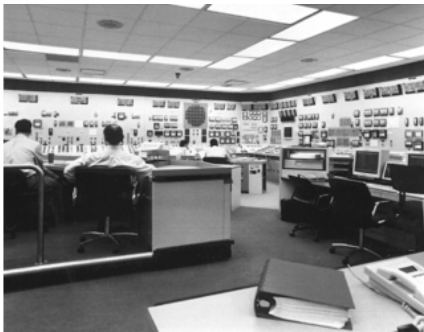
Control Room at a Nuclear Power Plant
