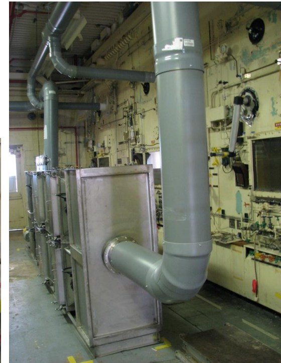
4507 Hot Cell Ventilation System
