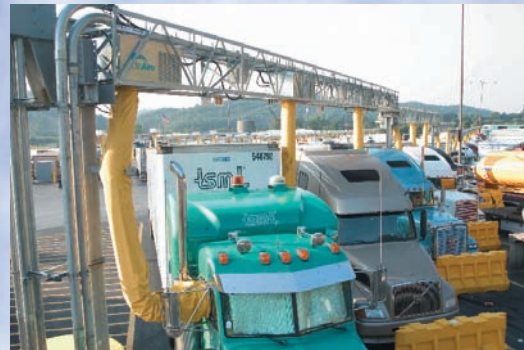
A simple window adapter makes this electrification system compatible with many models of long-haul trucks. Photograph courtesy of IdleAir.
