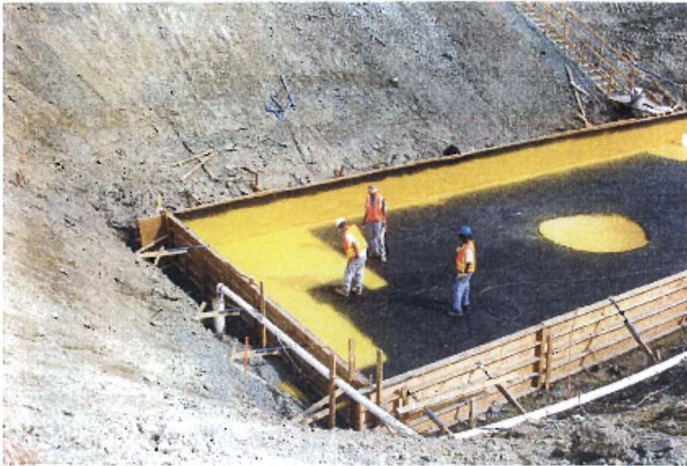
Above. Application of the 1 st coat of Integritank (yellow) on to the geotextile. The walls are sprayed first, followed by the slab, particularly at smaller sites, to ensure the material is cured at the applicators' entrance and exit points.
