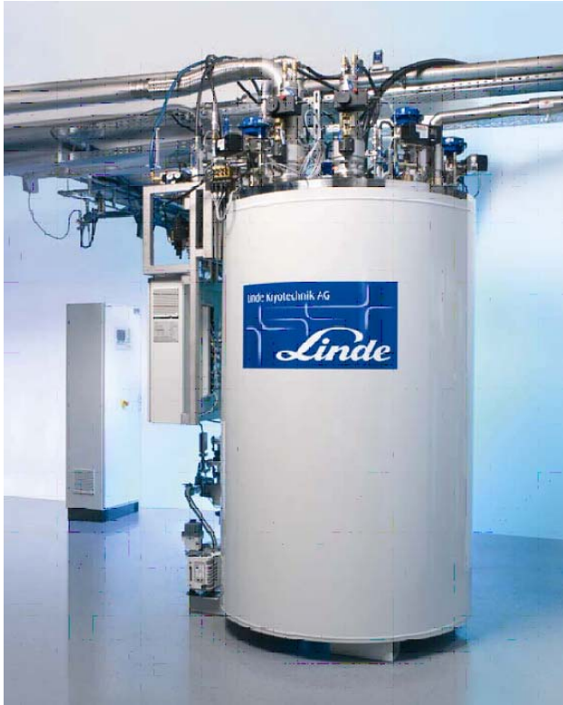
Figure 4.7.2. Typical R/L cold box.
