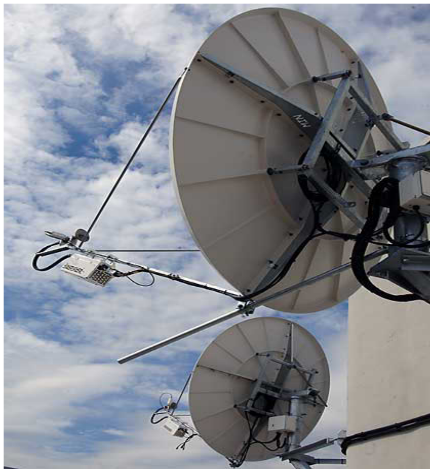
Figure 2: RM Satellite Network antenna on A-Tower IAEA, Vienna.
