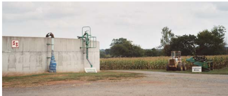
An animal waste storage tank (EPA OIG photo).
