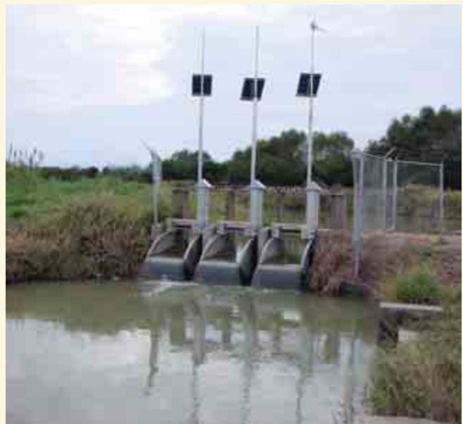
Replacement of manual gates with Rubicon standard programmable flume gate, Cameron County Irrigation District No. 2, TX, funded through the WaterSMART Grants program.
