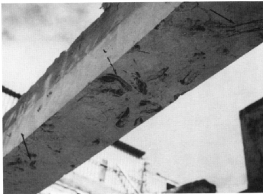
Figure 9. Shoe Sole Imprints on Bottom of Beam in Basement of HV Building.
