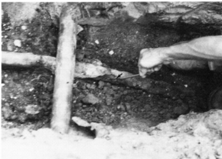
Figure 7. Location of Gas Leak from Inactive Gas Service Line under Arzuaga.
