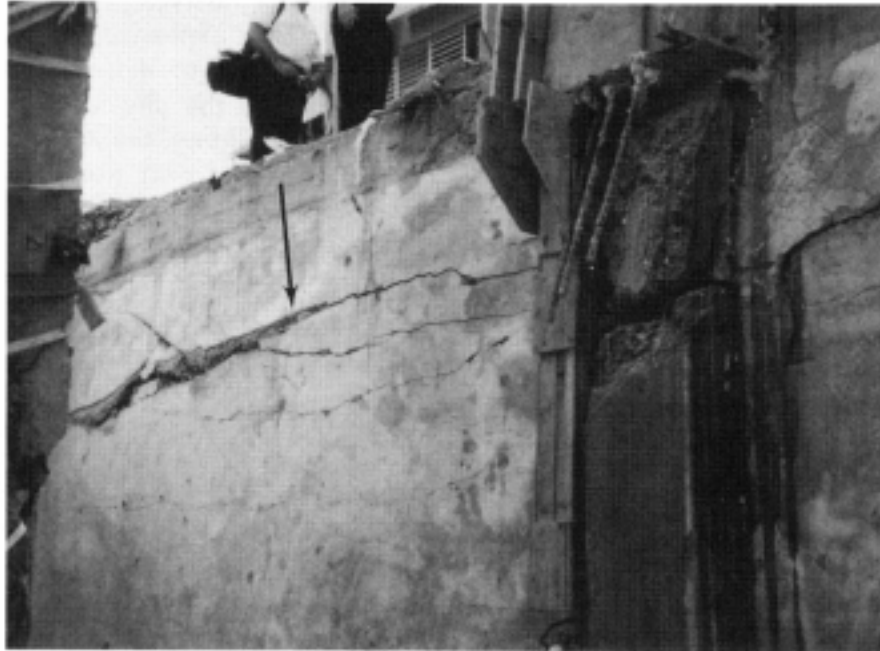
Figure 8. Major Crack in West Wall of Basement of HV Building.
