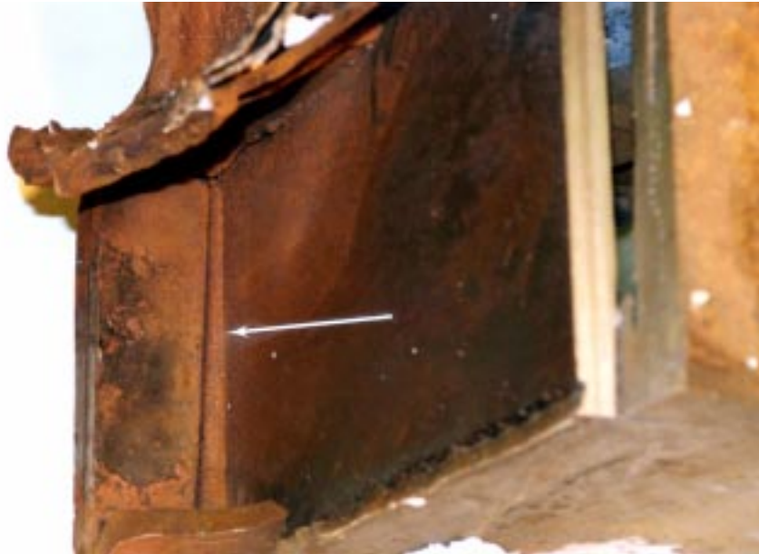
Figure 12. Arrow indicates threaded fastener at the joint welded and/or wedged in place
