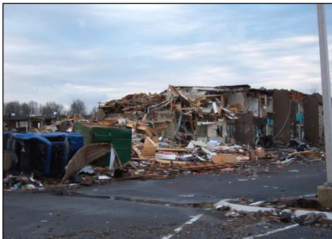
Figure 10. Damage to dormitories at Union University in Jackson, Tennessee. Courtesy of WFO Memphis.
