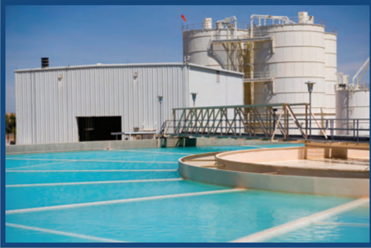
Solid Contact Reactor Clarifier at the Yuma Desalting Plant
