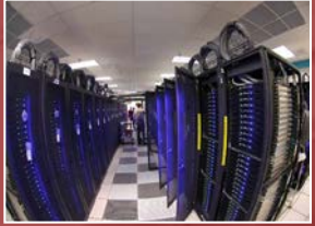
Red Storm HPC Facility
